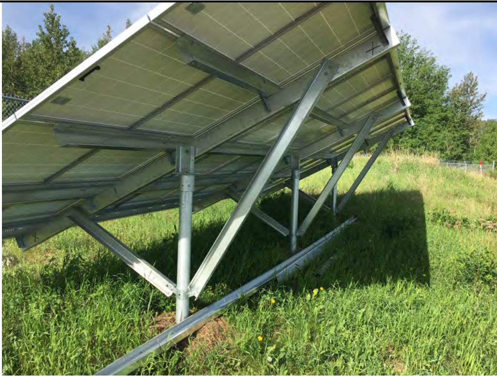
Plate 2: Demo racking currently on site
