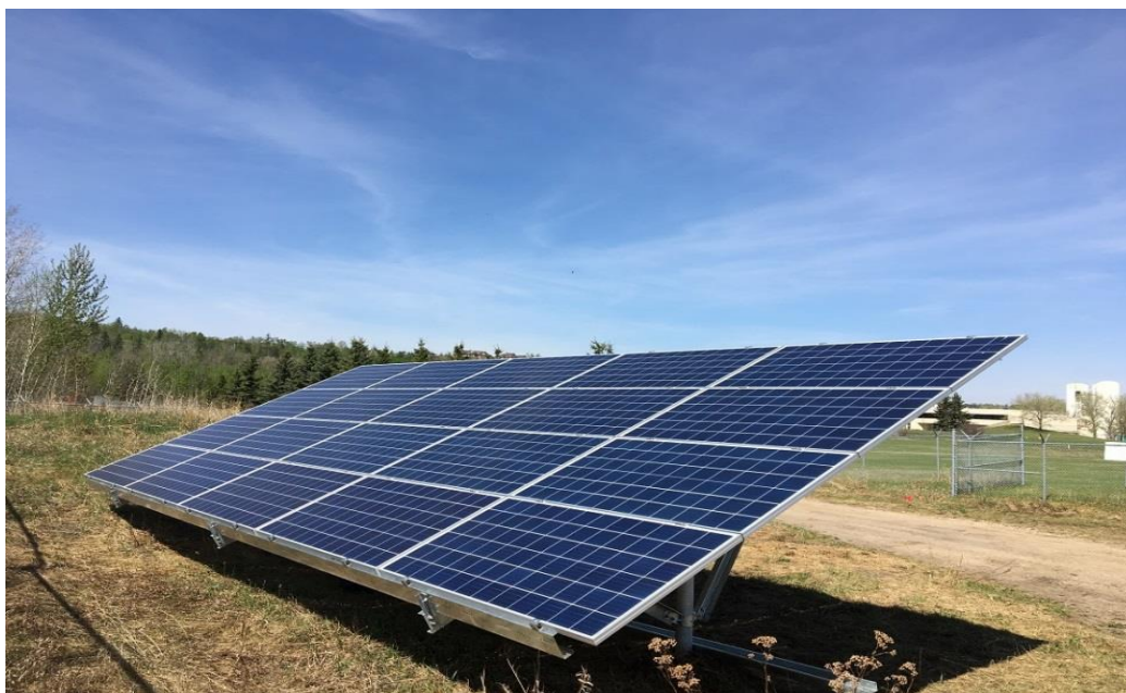
Figure 3.2-1 Solar Panel Demonstration at E.L. Smith Site
