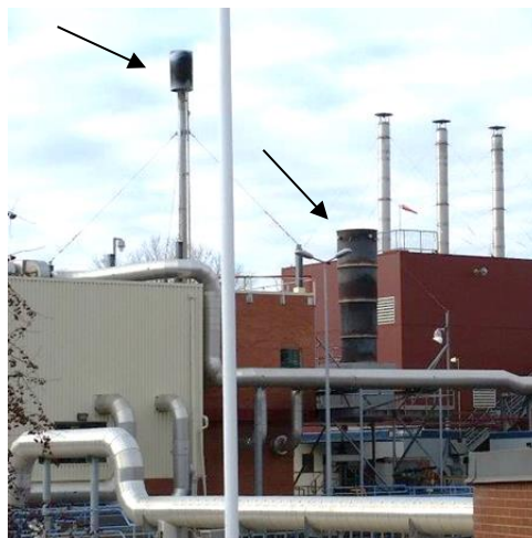
Figure 2.0-1 Flares at Gold Bar WWTP
