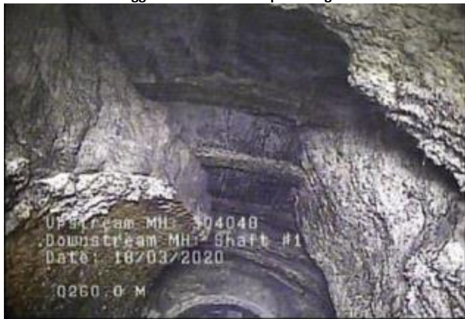
Figure 2.0-2 Duggan Tunnel - Close-up Missing Wall
