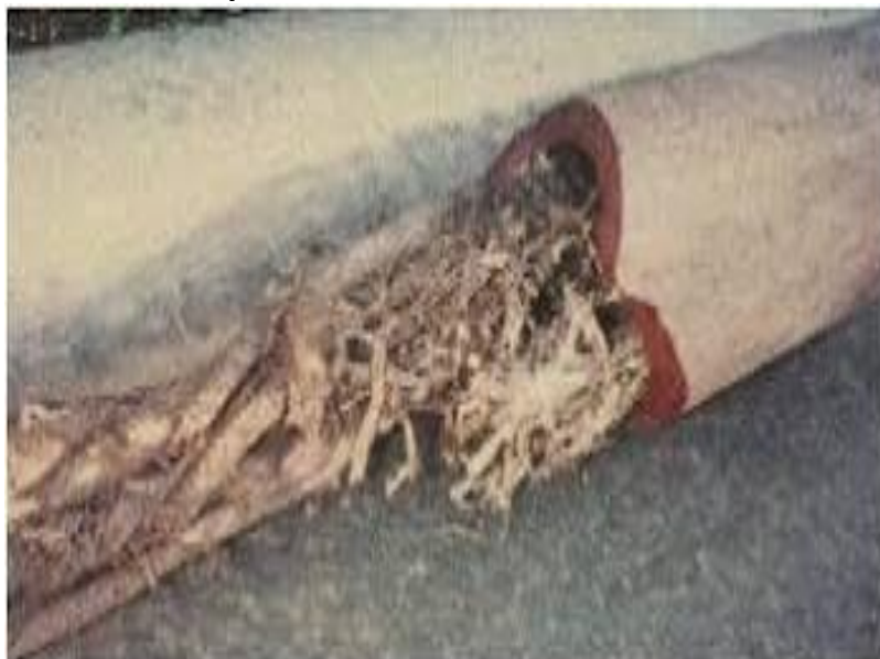
Figure 2.0-1 Sanitary Sewer Service Infiltrated with Roots
