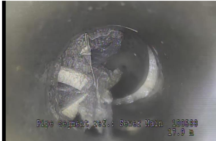
Figure 2.0-2 Broken Sanitary Service Line at Entry to Mainline
