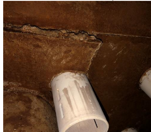
4. Separation of Transite Formwork
