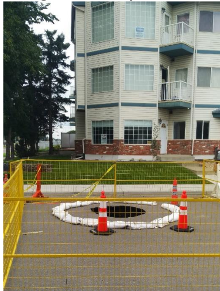
Figure 2.0-3 Image of Roadway Subsidence
