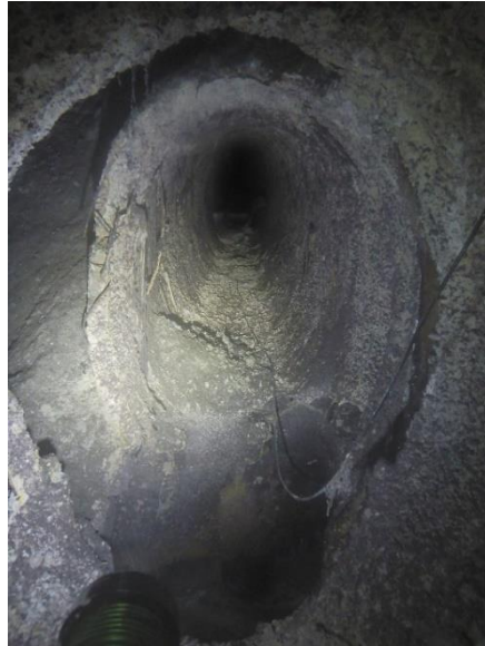
Figure 2.0-4 Large Void Upstream of Reach 49
