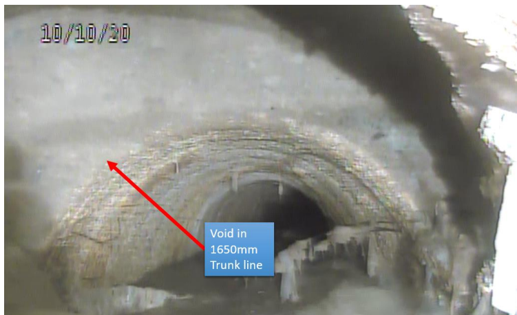
Figure 2.0-3 Void Inside 61 Avenue Trunk
