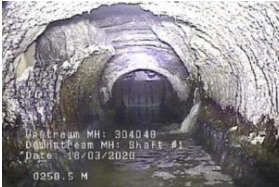
Figure 2.0-1 Duggan Tunnel - Missing Wall in the Trunk Sewer
