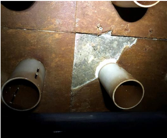
3. Spalled Piece of Transite Formwork
