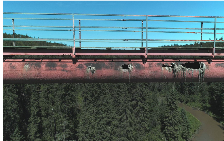
System rehabilitation investments include the repair and replacement of the Trestle 7 pipe, which failed due to internal corrosion. For more information on this project, see Appendix H-5.
