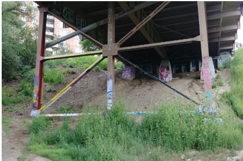
Plate 3.1. Erosion rills created by surface water runoff present on bridge abutment (02 August 2019)
