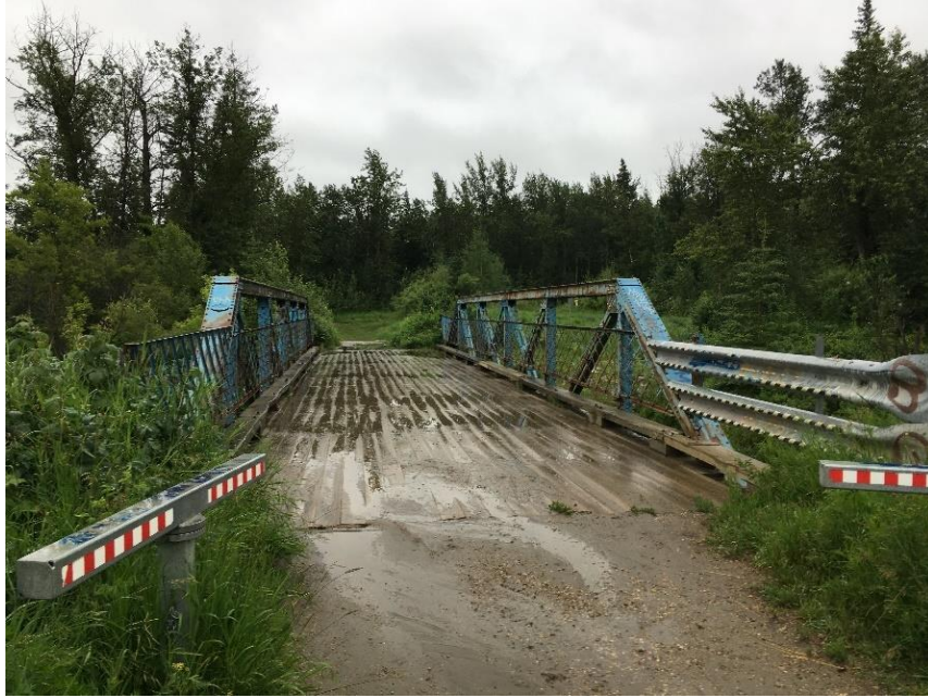
Plate 1.3. View south across bridge deck towards trailhead for McTaggart Sanctuary and trail to west up hill (19 July 2019).
