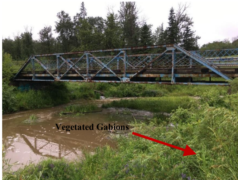
Plate 1.1. View to southwest of upstream side of pedestrian bridge crossing Whitemud Creek (prior to bank bioengineering) (19 July 2019).
