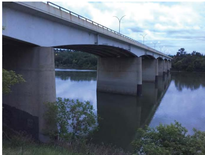
Plate 1.1. Groat Road Bridge over the North Saskatchewan River – view to south (08 June 2016)
