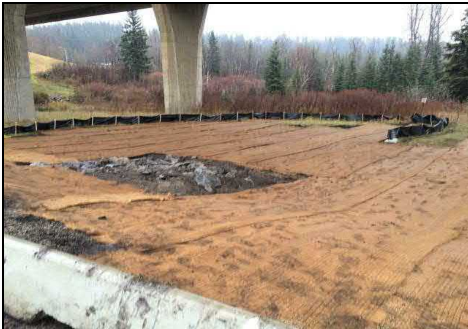
Photograph 10: The Site was re-seeded with a custom, native reclamation seed mix and then covered with erosion control blankets (October 25, 2016).
