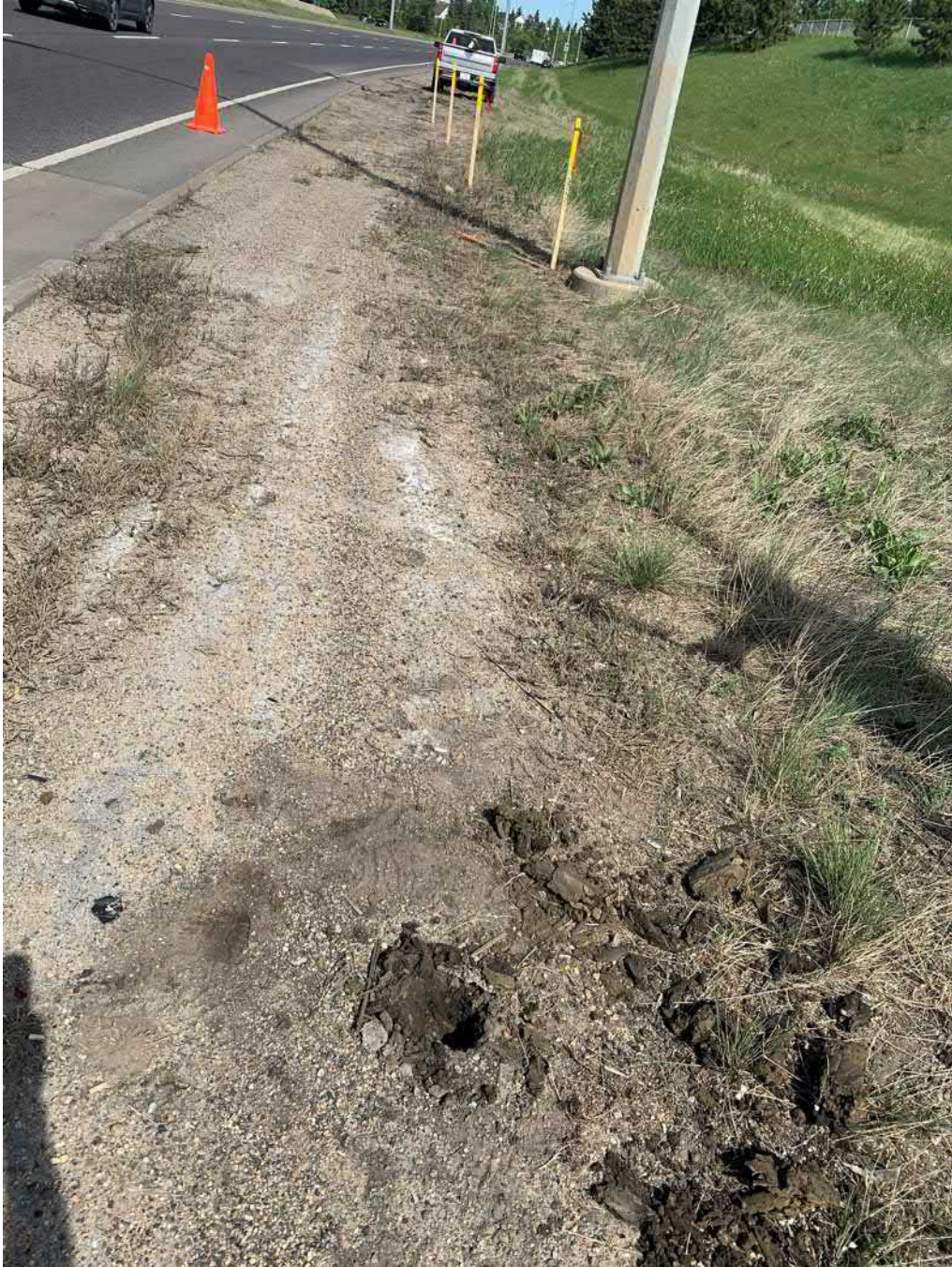
Photograph 5 – Salt staining at 21HA24 location, facing north along Whitemud Drive. June 2, 2021.
