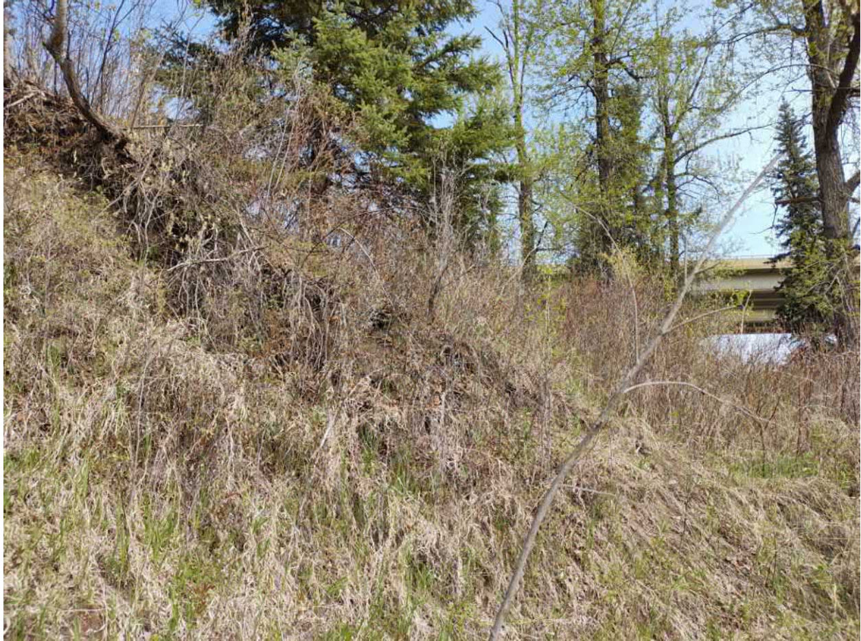
Figure 9. Small area of possible, highly weathered exposure. Note bridge deck at right of image. Photograph is taken looking north.
