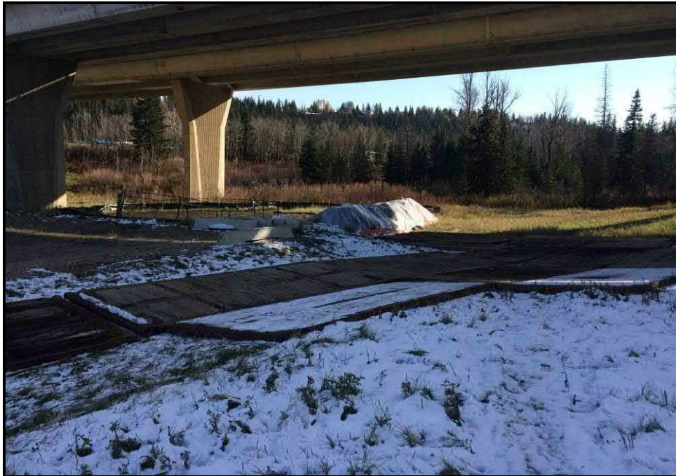
Photograph 5: Rig mats were installed from the gravel-surfaced parking lot to the Site, in order to provide access for loading of haul trucks and removal of the impacted soil (October 12, 2016).
