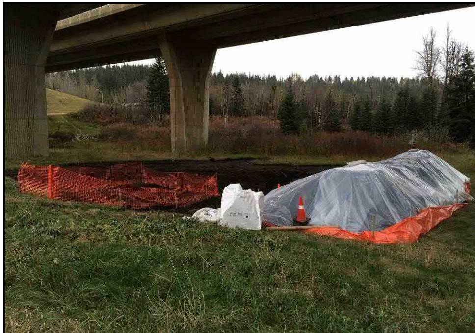
Photograph 4: Impacted soils were contained in a poly-lined cell onsite for future disposal once landfill approval was granted (October 7, 2016).
