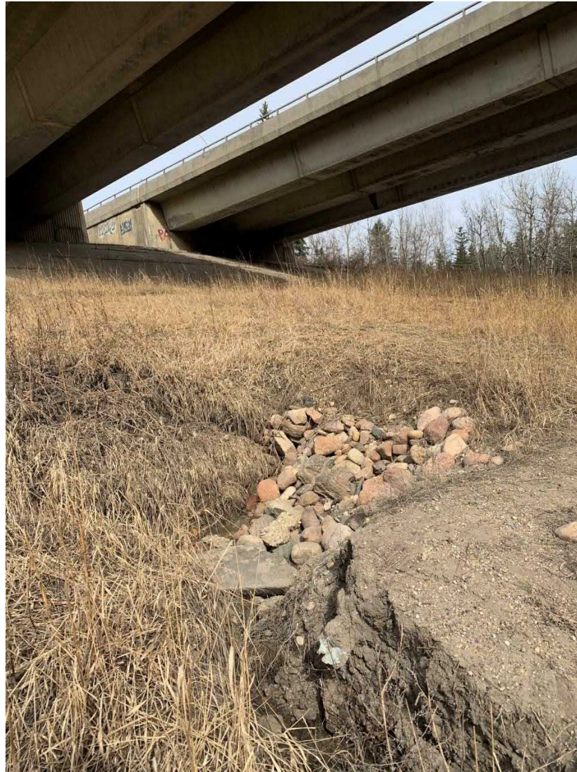
Photograph 6 – Facing northwest toward RVB, soil erosion and debris. April 22, 2020.
