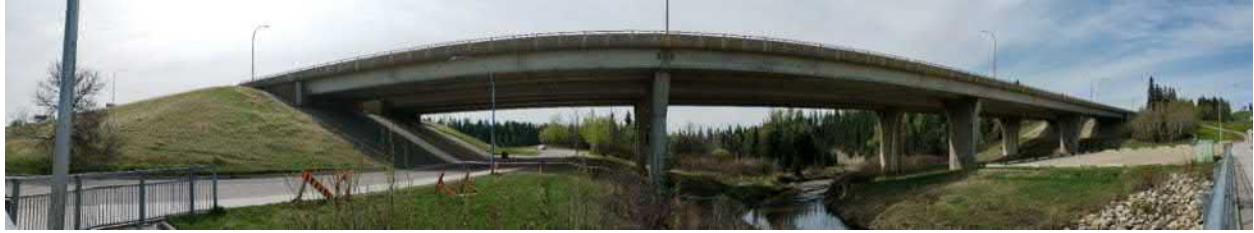
Figure 12. View of the Rainbow Valley Bridges, looking south. Note graded, vegetation covered slopes next to the bridges and lack of exposed bedrock in the area.
