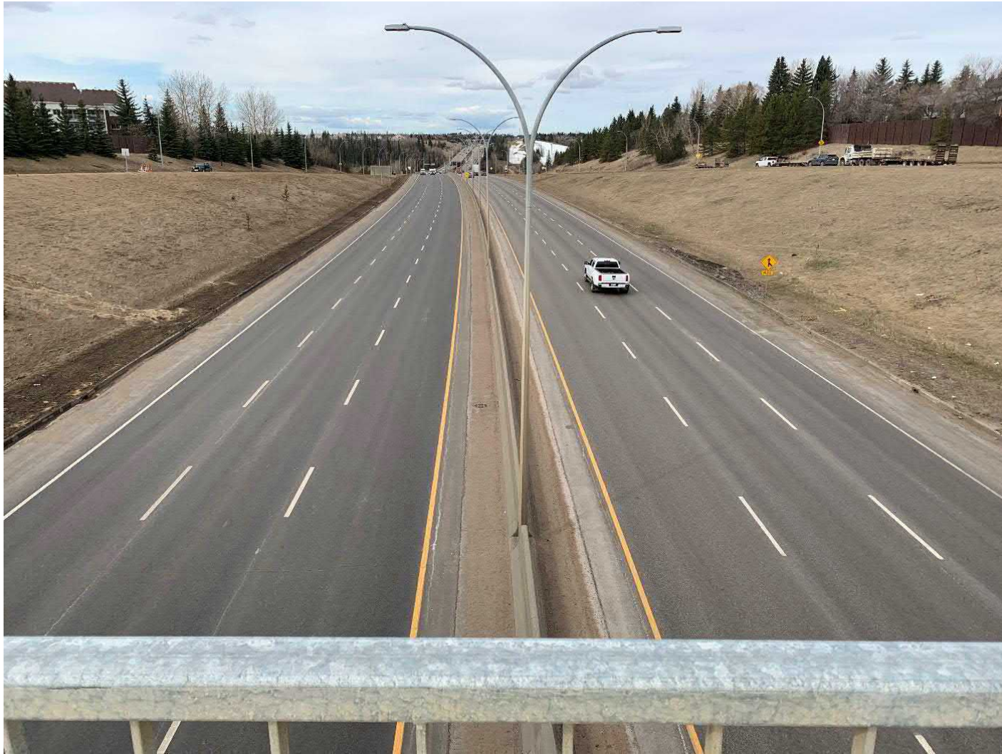
Photograph 9 – Facing west from 122 Street Bridge, salt staining on WMD. April 22, 2020.
