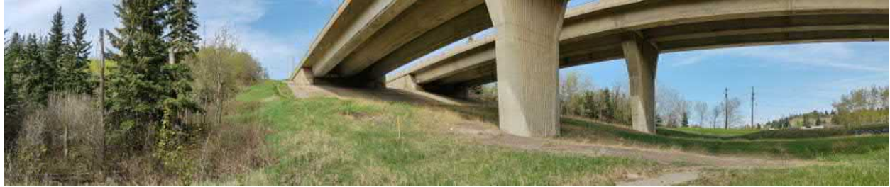
Figure 11. View from Whitemud Creek, looking northwest, of the slopes underneath the Rainbow Valley Bridges. Note the small patches of exposures in the centre of the image; these patches are all reworked deposits, likely from the original construction of the bridges.
