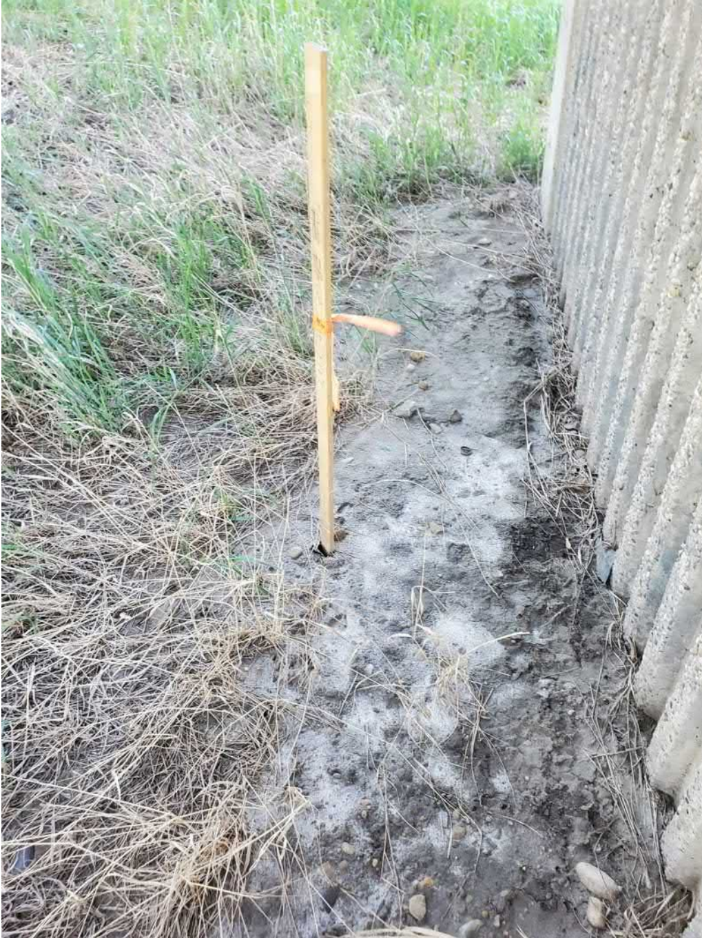
Photograph 3 – Salt staining at 21HA19, adjacent to pier below Rainbow Valley Bridges. June 4, 2021.
