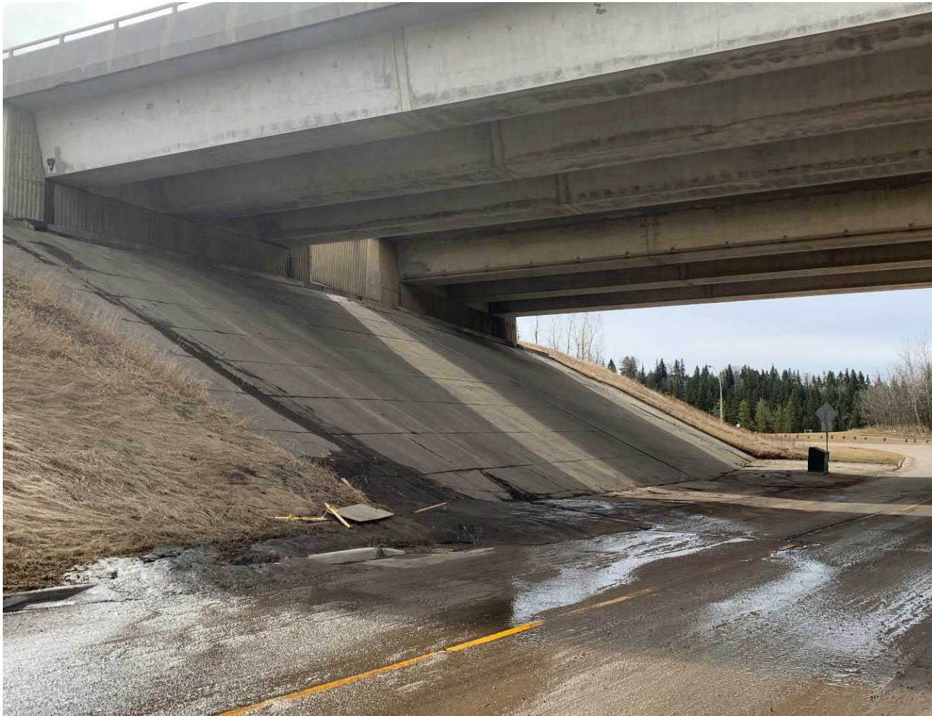
Photograph 7 – Facing southeast toward RVB, catch basin, box containing gravel, and cracks in lower concrete. April 22, 2020.
