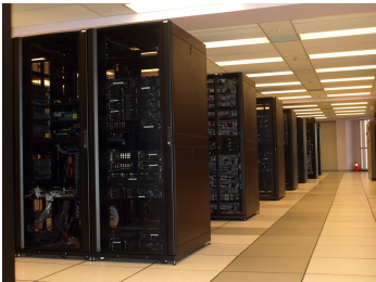
Technology Equipment Assets in the City of Edmonton Data Centre
