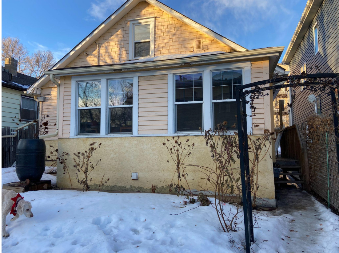
South (rear) elevation, looking north (south elevation is not subject to designation, provided for context).
