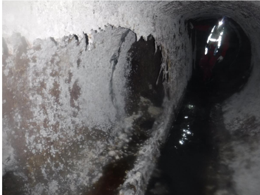
Figure 2.4.5-4 Sanitary Drop Pipe 116 Street and 108 Avenue
