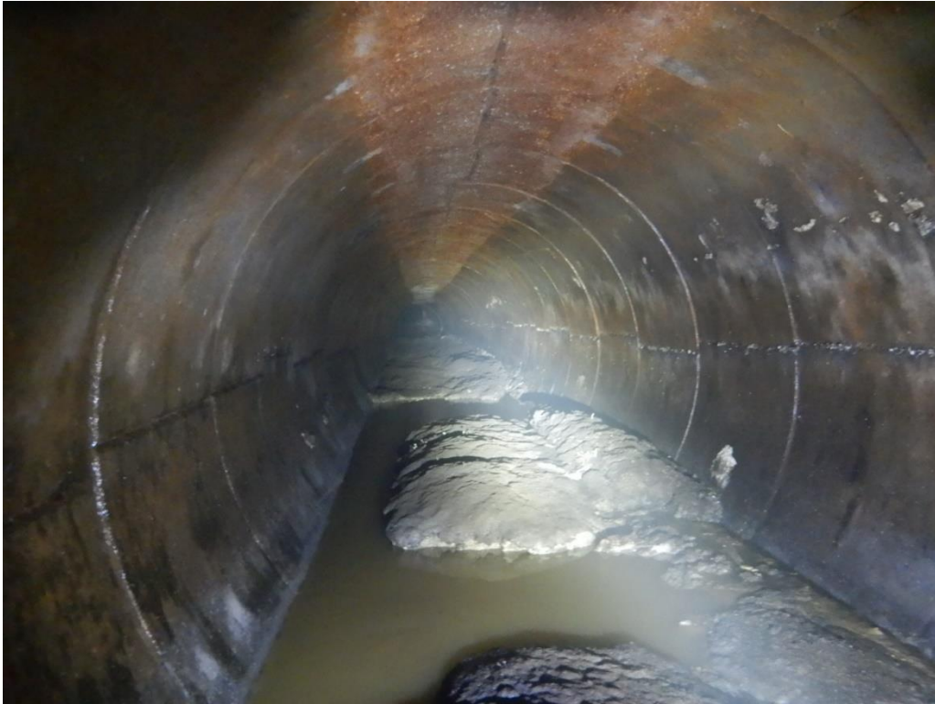
Figure 2.4.5-6 NL1 Tunnel solid accumulation
