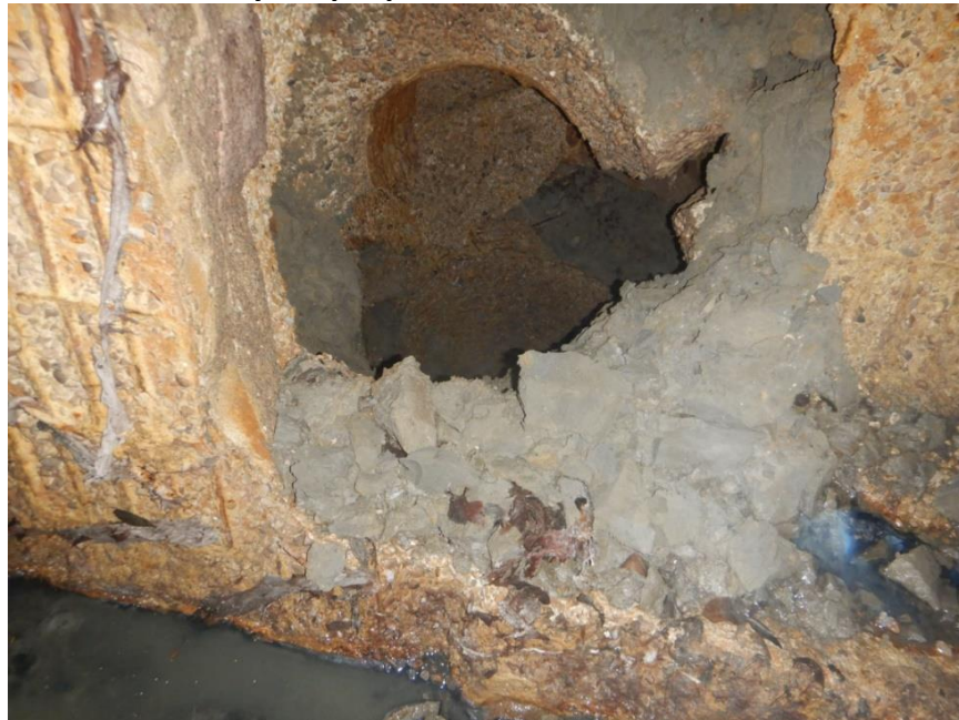
Figure 2.4.5-3 Sanitary Drop Pipe 116 Street and 108 Avenue
