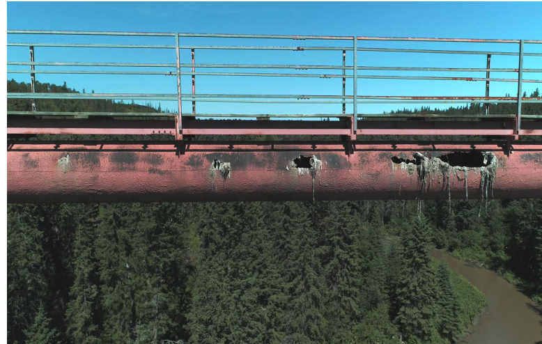
System rehabilitation investments include the repair and replacement of the Trestle 7 pipe, which failed due to internal corrosion. For more information on this project, see Appendix H-5.
