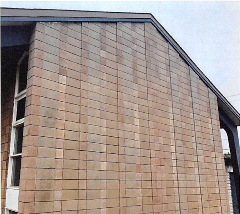
East Elevation - Concrete Block Masonry Units Arranged to Create Patterns and Textures
