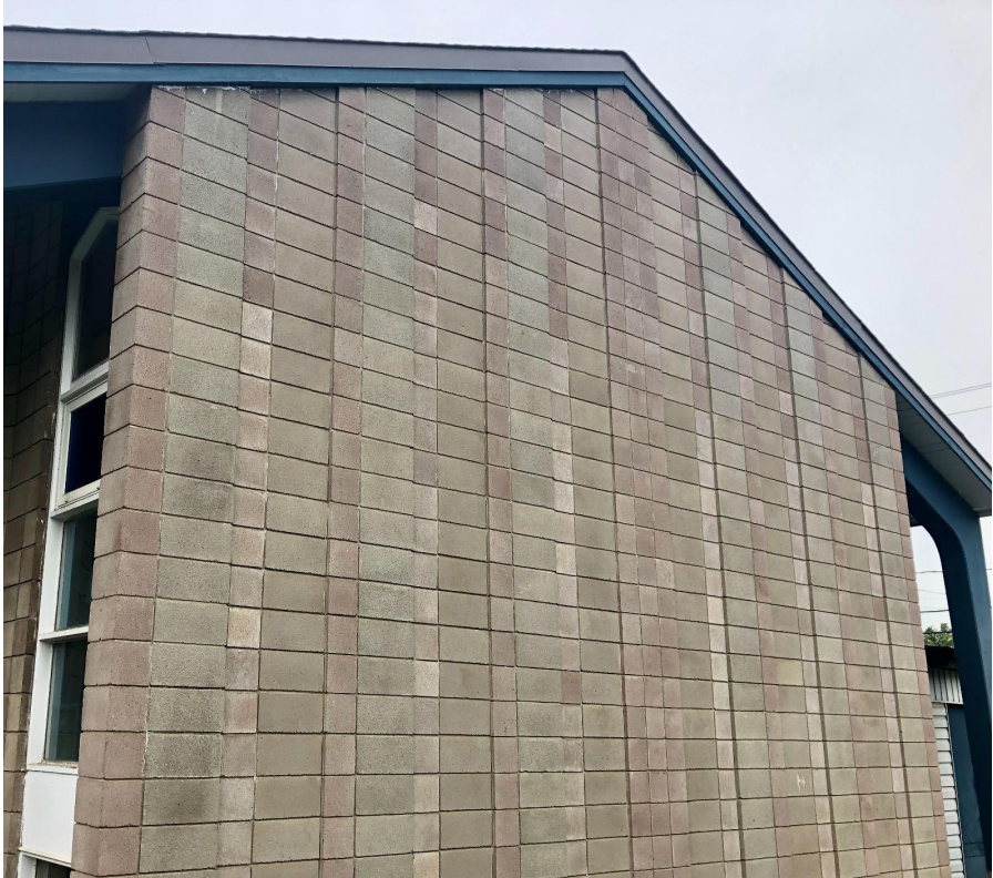
East Elevation, 2022 - Concrete Block Masonry Units Arranged to Create Patterns and Textures
