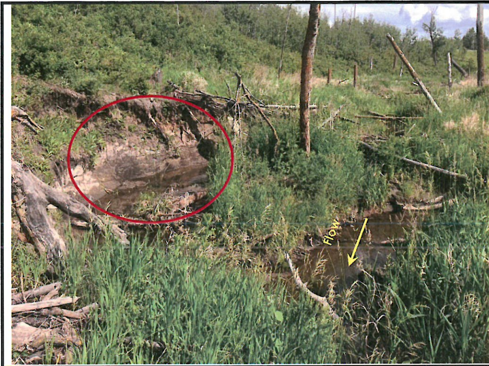
Photo 11: Looking upstream (south) at upstream of proposed crossing. Note lateral bank erosion.
