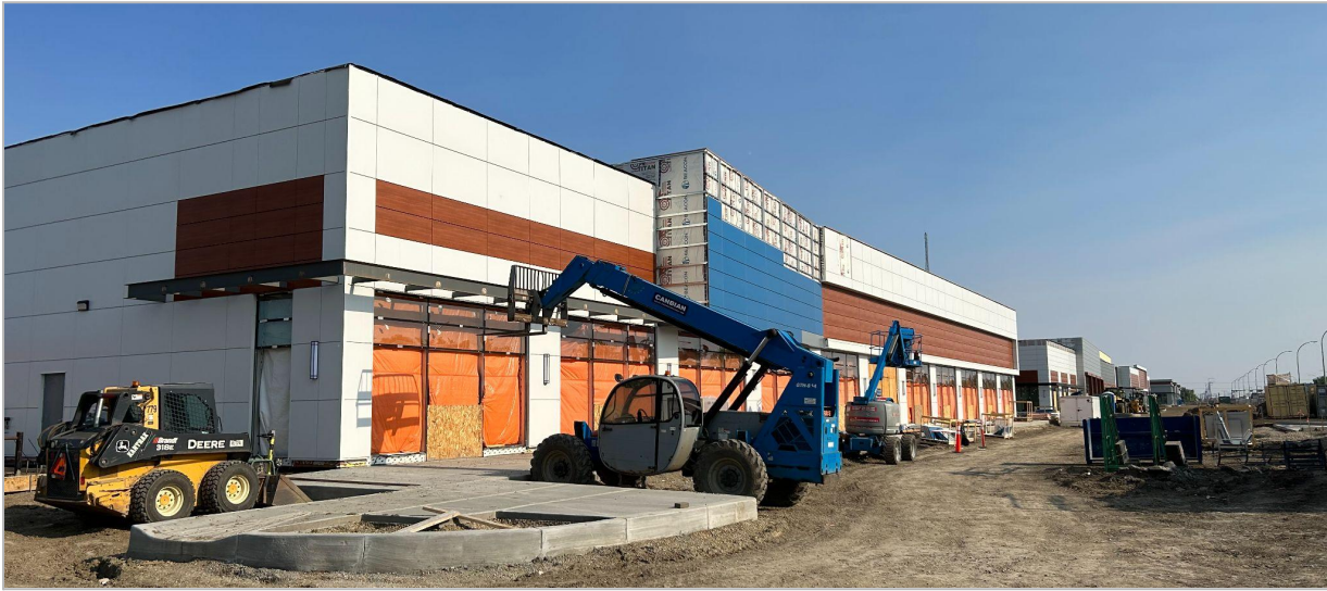
View of the site looking southeast from Gateway Boulevard NW and 37 Avenue NW
