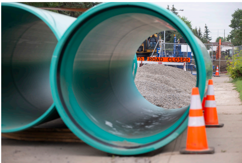
PVC Sewer Pipes
