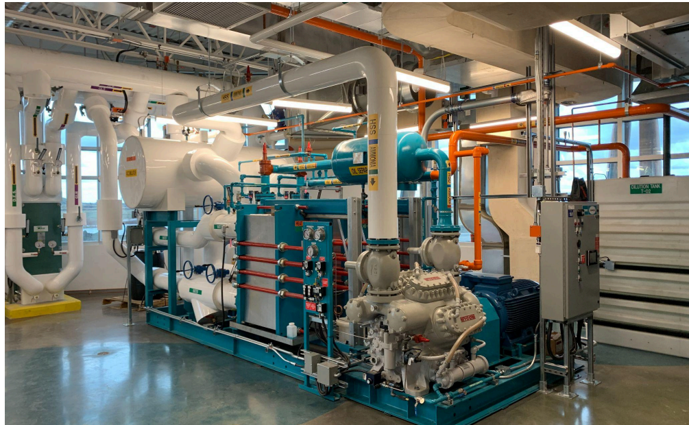
A second heat pump installed in late 2023 increases the District Energy Sharing System's existing capacity so it can continue meeting Blatchford's heating and cooling needs as the community expands.
