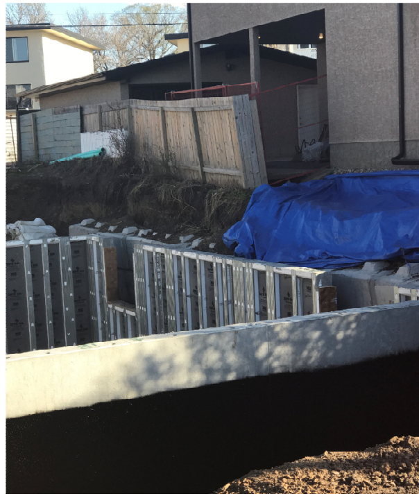
Impacts to adjacent structure
