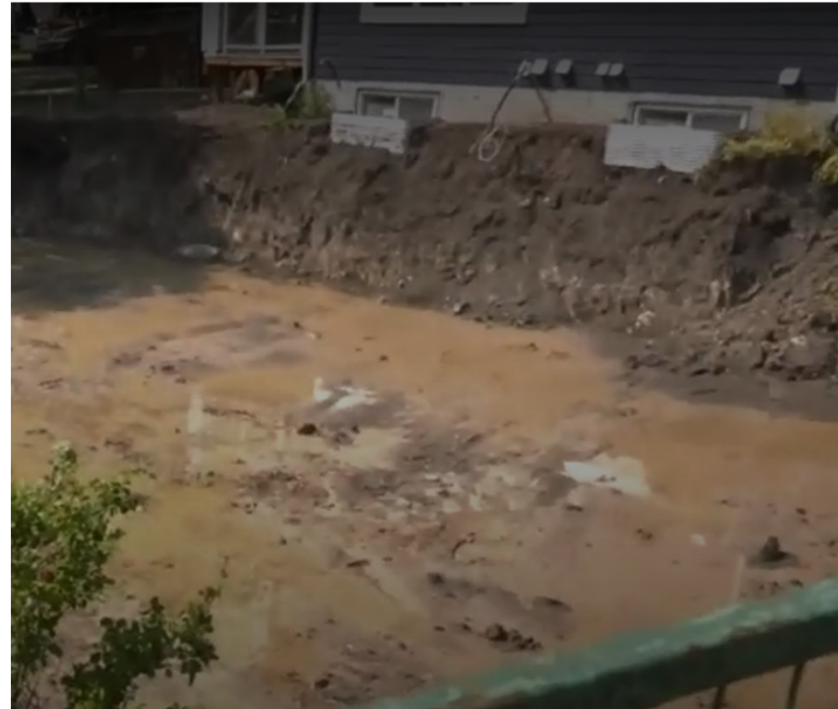
Water accumulation & impacts to new infill home
