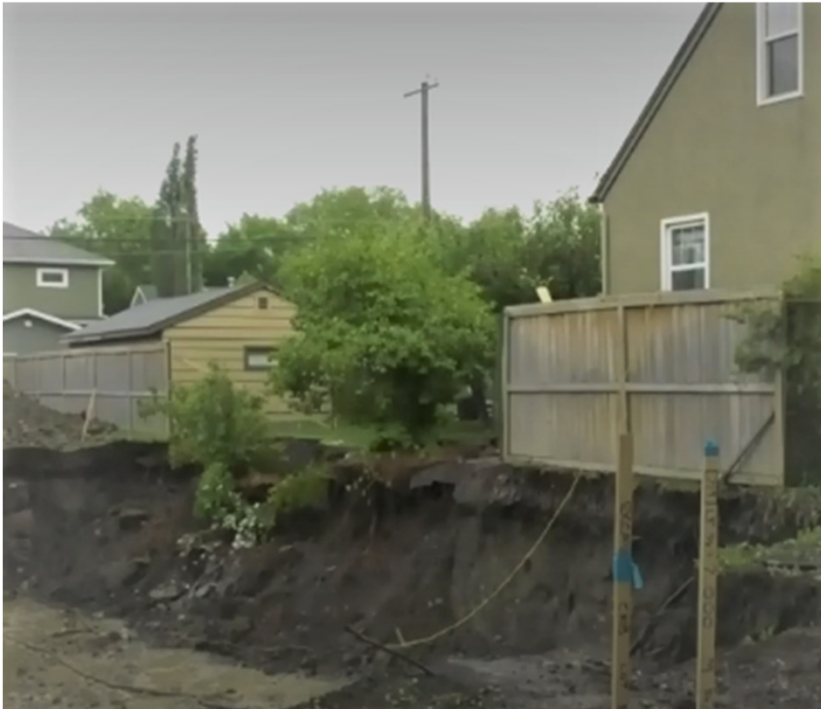
Failure next to mature development
