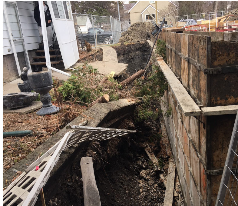
Impact to adjacent structure & side yard
