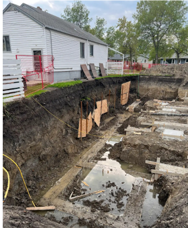
Excavation failure & heavy rain
