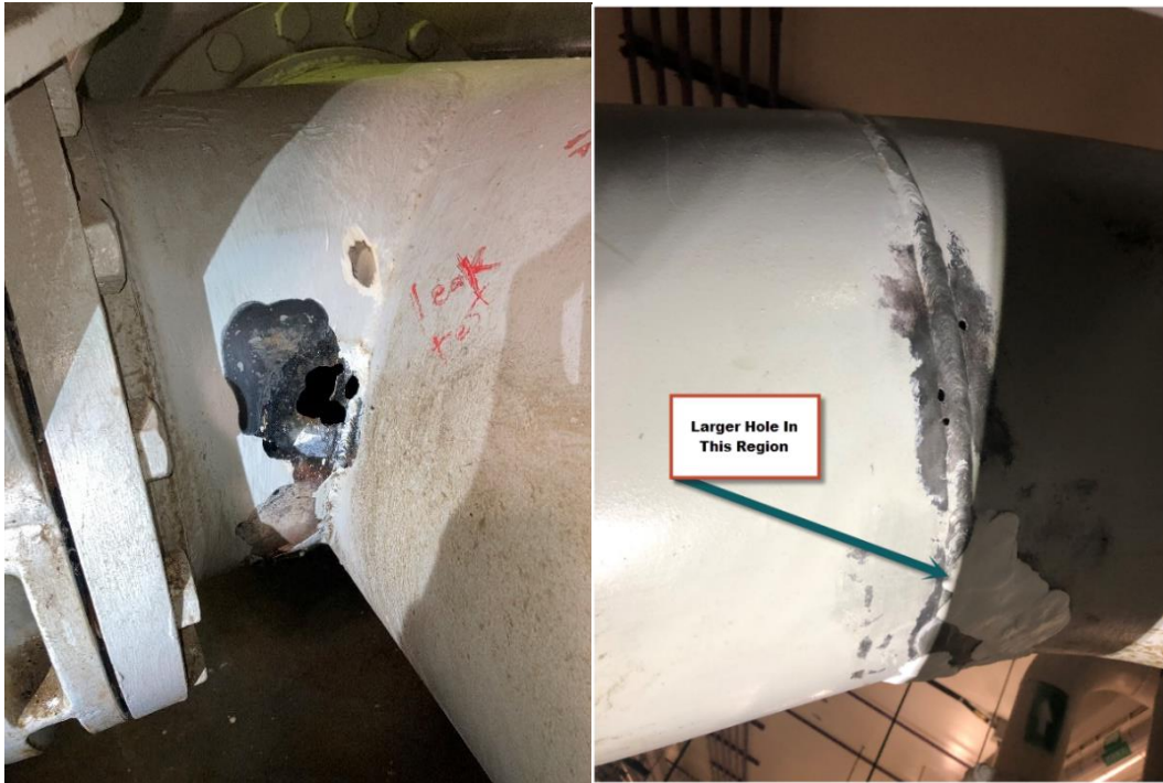
Figure 3.0-1 Holes in RAS/WAS Piping System
