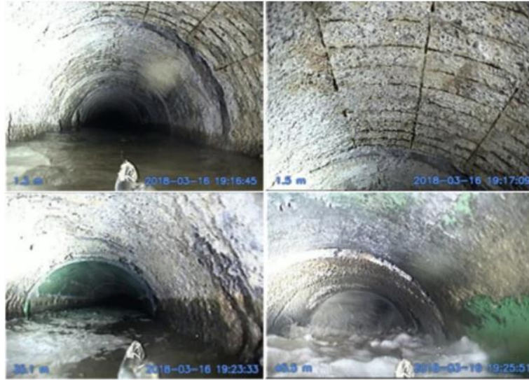
Figure 3.0-1 Deterioration of Small Trunks
