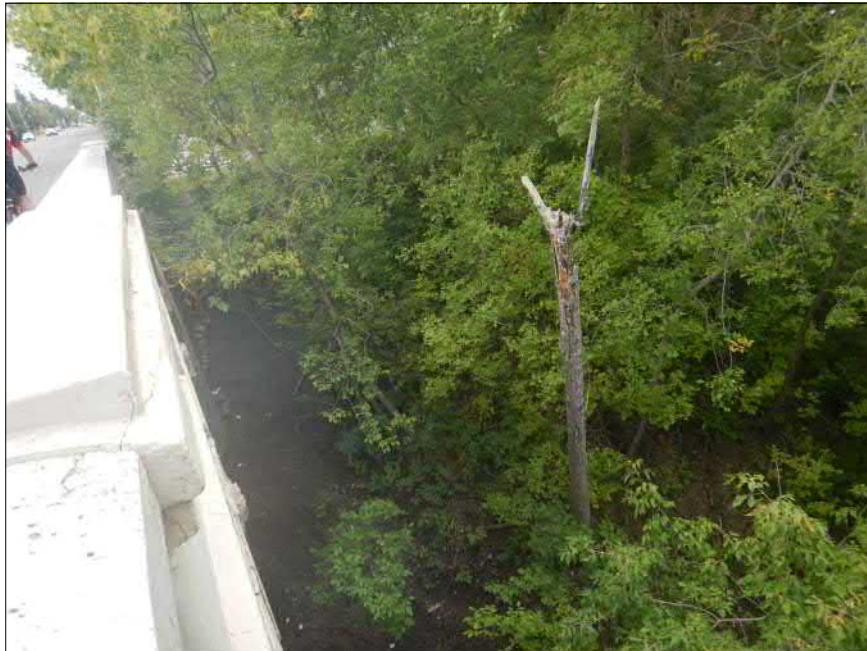
PHOTO 6 EROSION ON WEST RAVINE SLOPE NORTH OF BRIDGE
