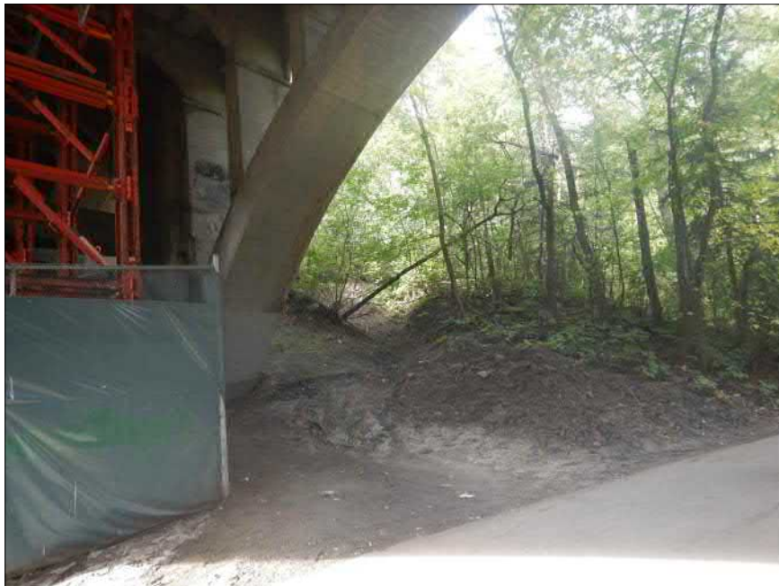
PHOTO 8 EROSION ON WEST RAVINE SLOPE NORTH OF BRIDGE
