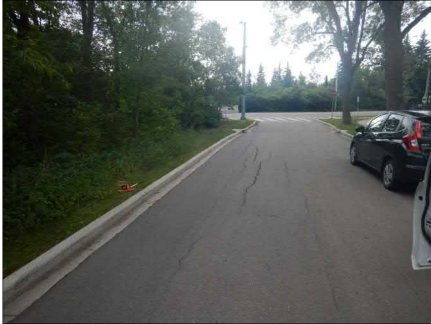
PHOTO 1 CATCH BASIN AND CRACKING ON CHURCHILL CRESCENT LOOKING SOUTH TOWARDS 102 AVENUE
