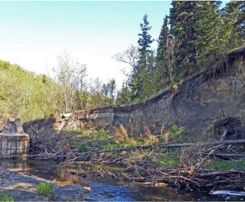
Erosion of Millcreek Ravine, 2024 that is related to increased development imperviousness and increasing impacts of climate change & extreme rainfall events. Further damage must be mitigated.
