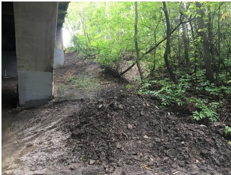
Figure 3-1 View of active landslide northwest of Wellington Bridge
