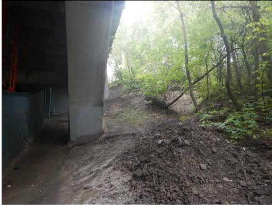
PHOTO 7 EROSION ON WEST RAVINE SLOPE NORTH OF BRIDGE
