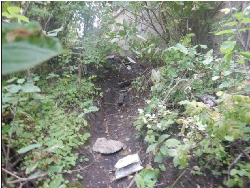
PHOTO 10 EROSION ON EAST RAVINE SLOPE NORTH OF BRIDGE
