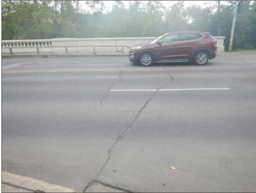
PHOTO 9 DIAGONAL CRACKING ON 102 AVENUE IN WEST ABUTMENT AREA
