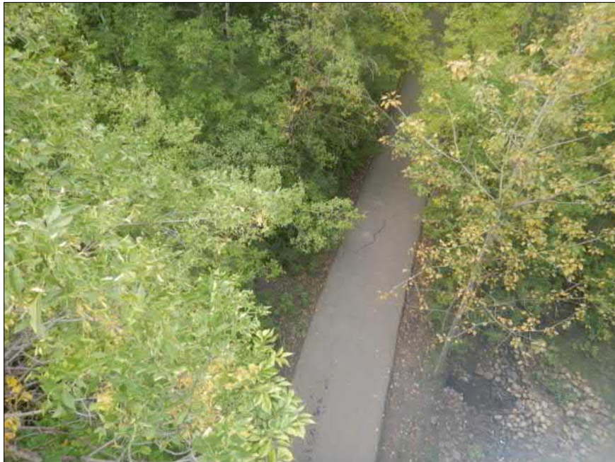
PHOTO 4 SURFACE CRACKING ON MULTI-USE TRAIL BETWEEN RETAINING WALL AND BRIDGE
