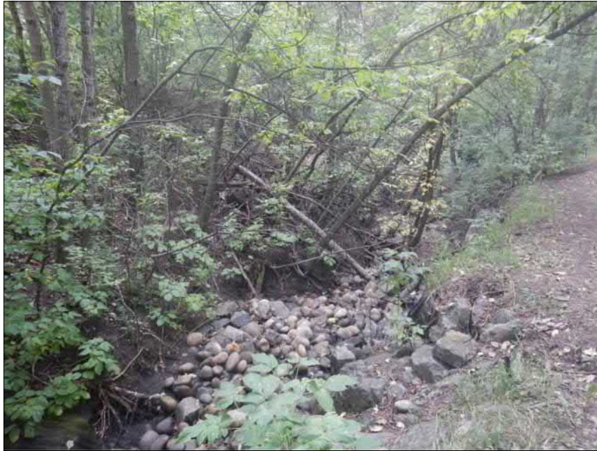
PHOTO 11 DRAINAGE CHANNEL DISTURBANCE EAST OF MULTI-USE PATH SOUTH OF BRIDGE
