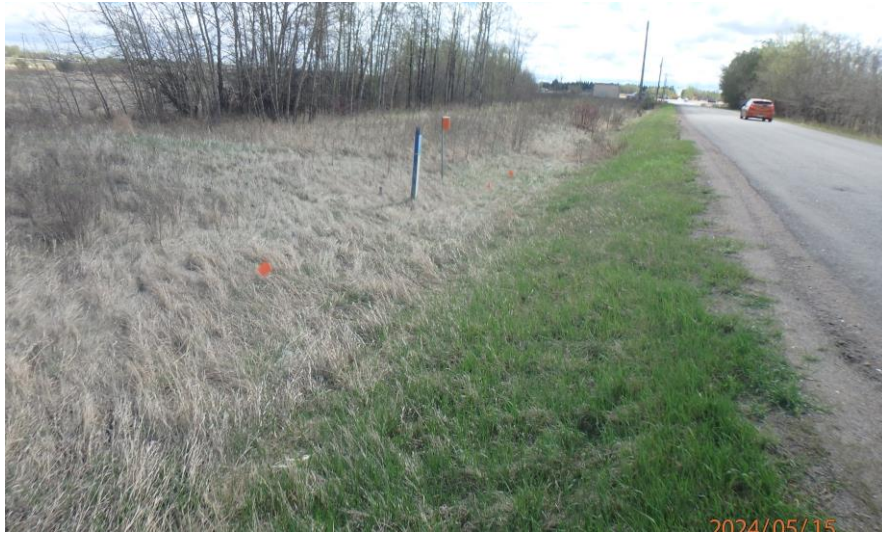
Photo plate #13: View of road side slope, south of the bridge (May 15, 2024) (12U 343470.28 m E/ 5948381.63 m N)
