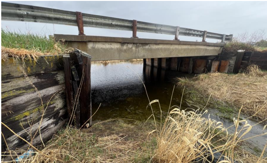
Photo plate #15: Photo of bridge, looking upstream, showing large scour hole followed by small channel width downstream (May 16, 2024).
