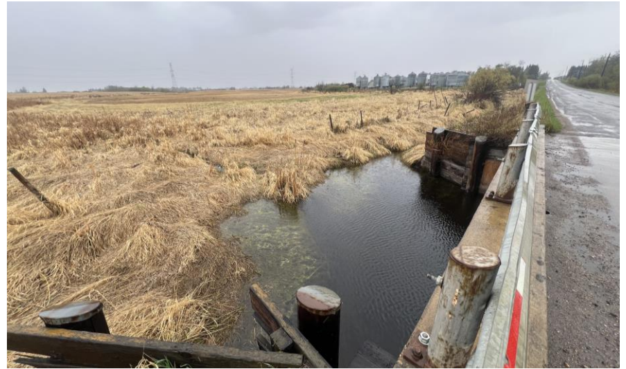
Photo Plate #14: View upstream from bridge, showing drainage entering from the west (May 16, 2024)
