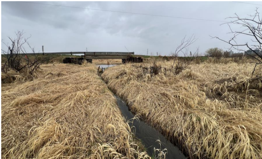
Photo plate #19: view upstream towards bridge showing constrained channel width (May 16, 2024).
