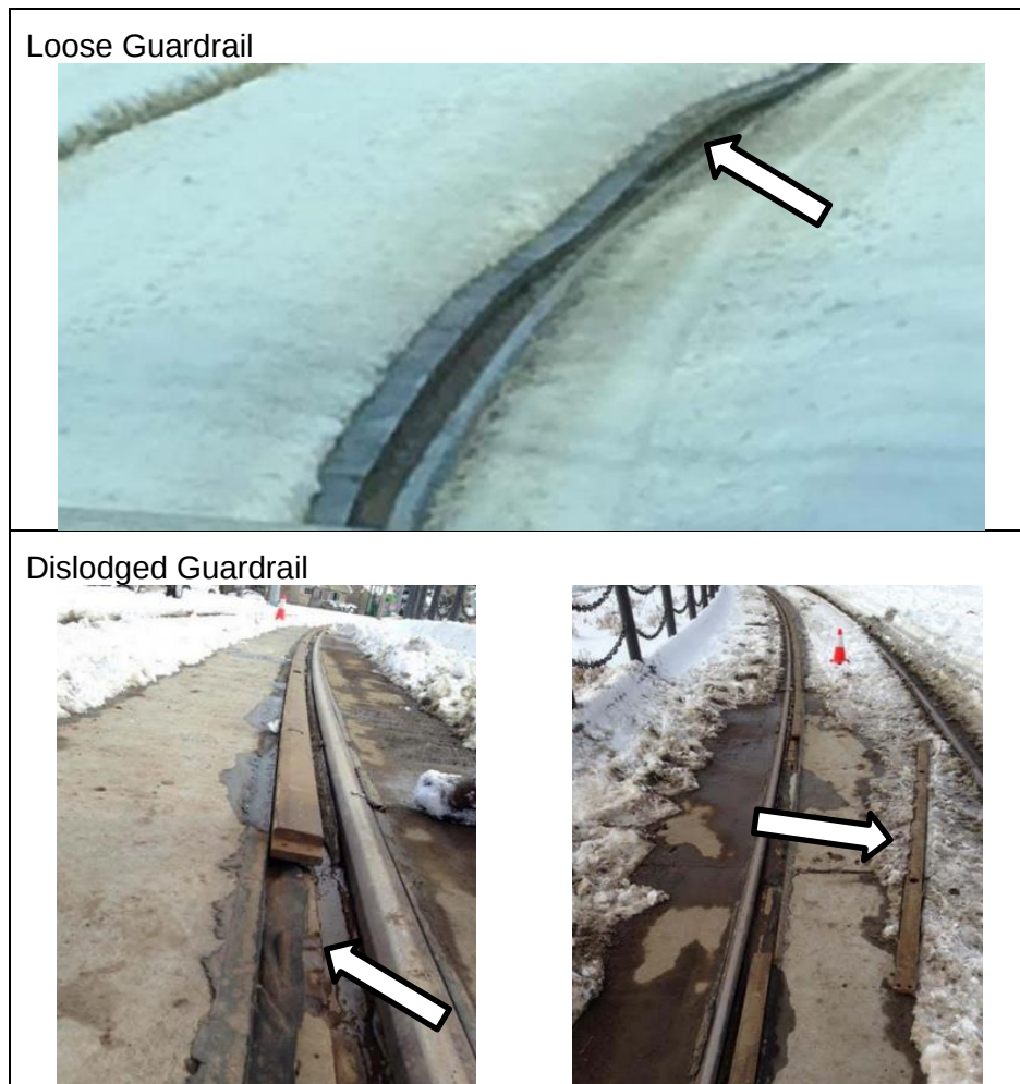
Figure 3 – Guardrail Track Issues
