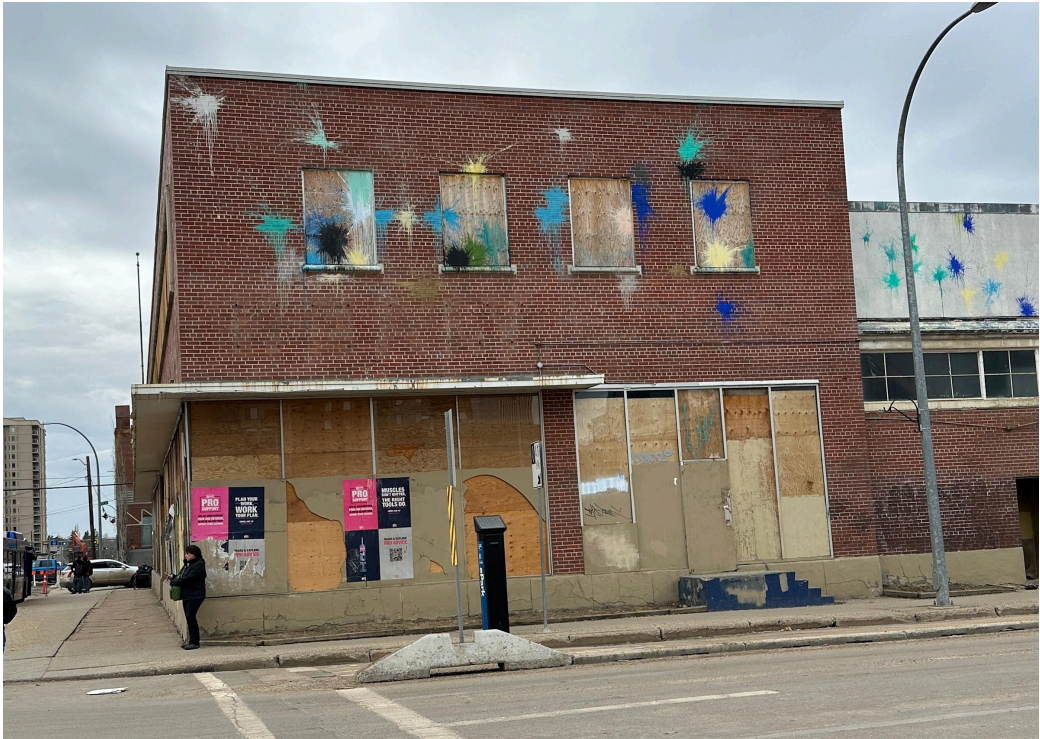
View of side (east) elevation, looking west from 106 Street NW. The lower height addition to the right of the two-storey 1947 building is not part of the designation and will be demolished.
