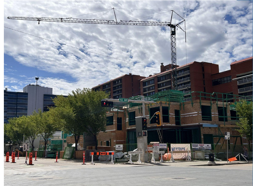
Lotus Park - IIF-supported development by Westrich Pacific, located at 108 Street and 102 Avenue
