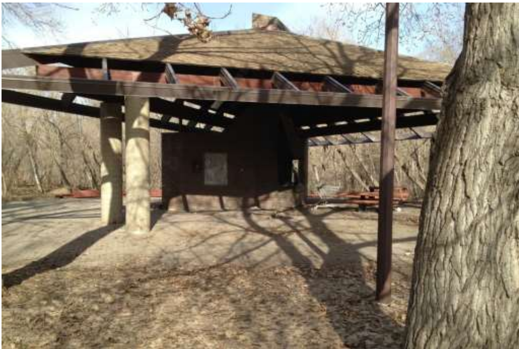
Plate 2.4. Derelict picnic shelter and grounds in HMEP (April 2013).
