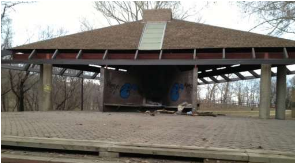
Plate 5.8. The picnic shelter and hard surface appear to be in disrepair and public fireplaces installed as part of the picnic shelter structure have been boarded over (April 2013).
