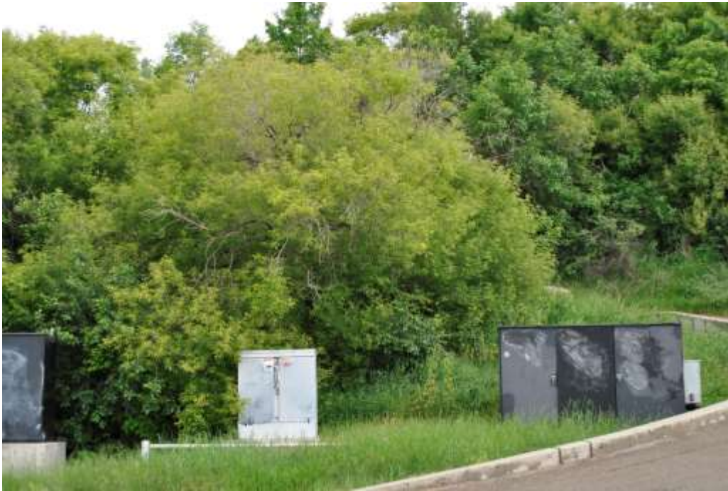
Plate 4.15. Several utility panels/boxes are located along the vehicle access road turnaround, looking north.
