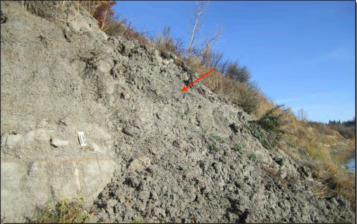
Figure 14. View looking east along north valley wall of North Saskatchewan River showing exposed bedrock from the Horseshoe Canyon Formation. Slide scar (→).
