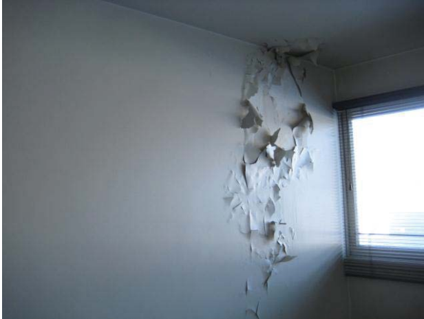
C3010.11 – Interior Wall Painting Location – Stairwell To Basement Component – Deteriorated Finish Deficiency – Study & Repair
