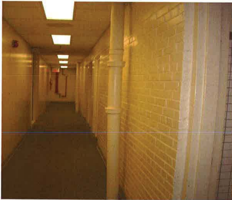
Photo 1: Suspect asbestos-containing Bell and spigot joint packing associated with cast iron waste/drain pipes (found in the corridor (Rm. 29)).
