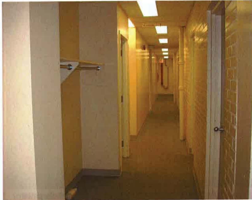
Photo 4: Asbestos-containing drywall joint compound as found in the corridor (Rm. 29).
