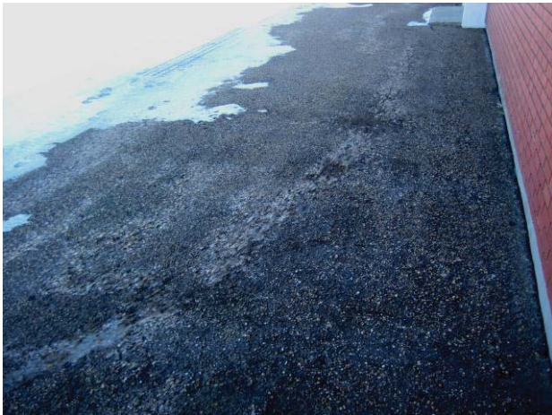
G2010.02.02 –Flexible Pavement Roadway (Asphalt) Location – Access Lane (West Elevation) Component – Asphalt Surfacing Deficiency – Deteriorated & Past Maximum EUL
