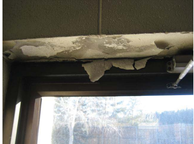
C3010.11 – Interior Wall Painting Location – Apparatus Floor Component – Deteriorated Finish Deficiency – Study & Repair
