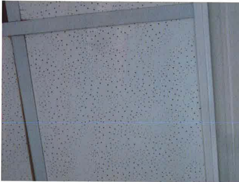
Photo 6: Asbestos-containing 2'x4' ceiling tile (pinhole pattern) as found in the side entrance (Rm. 27).
