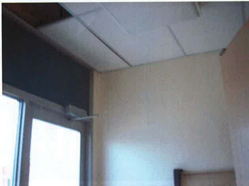
Photo 5: Asbestos-containing 2'x4' ceiling tile (pinhole pattern) as found in the side entrance (Rm. 27).
