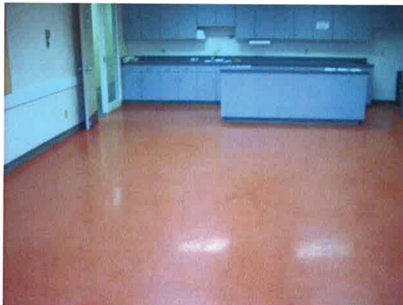
Photo 3: Asbestos-containing 12"x12" vinyl floor tile (Red) as found in the lunch room (Rm.28).
