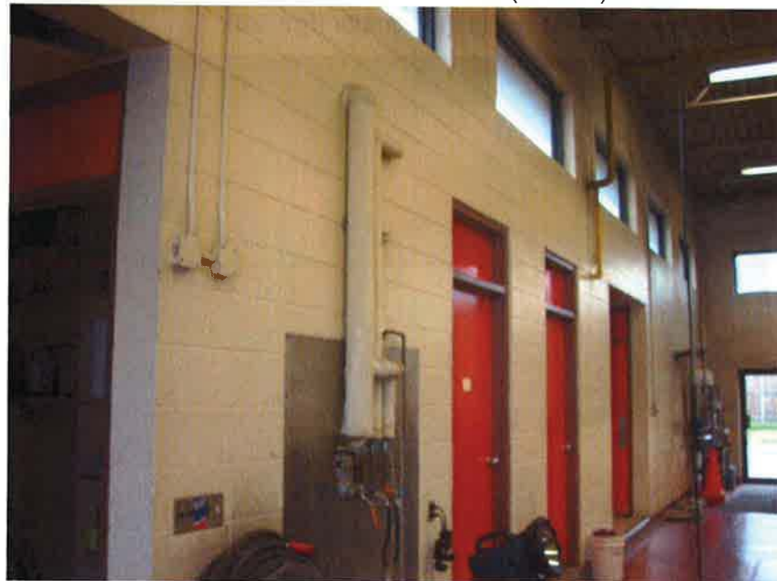
Photo 7: Asbestos-containing pipe parging insulation as found in the apparatus floor (Rm. 47).
