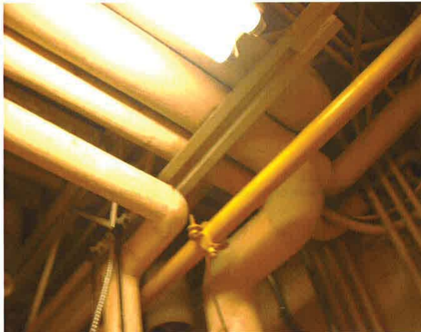
Photo 8: Asbestos-containing pipe parging insulation as found in the mechanical room (Rm. 53).
