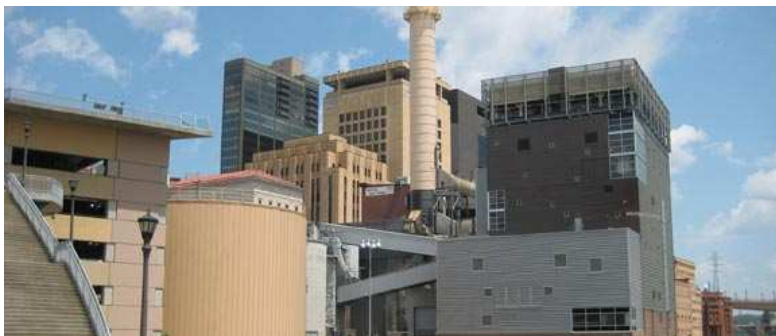
District Energy System St. Paul •Bio-Mass Fueled •Hot Water District Heating 31.8 million sqft
