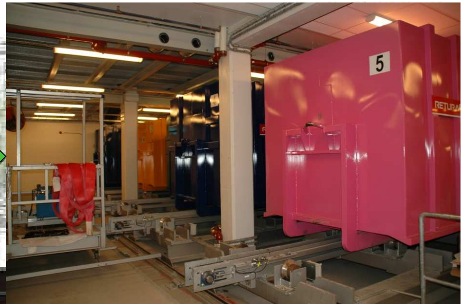
Underground Vacuum Collector
