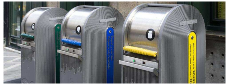
Pneumatic Waste System •Over 600 installations in 20 countries •Quartier des Spectacles Montreal •La Cite Verte, Quebec
