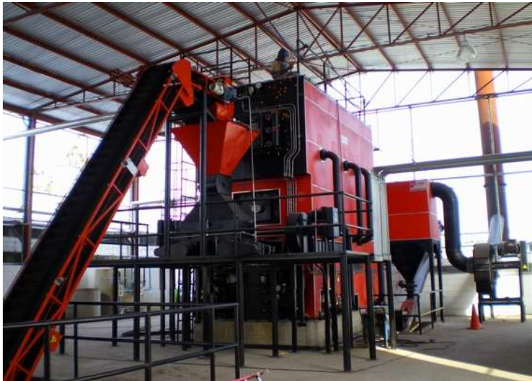
Wellons Biomass Thermal Fluid Heater •30 Years in Business in Western Canada •Hundreds of Industrial Installations
