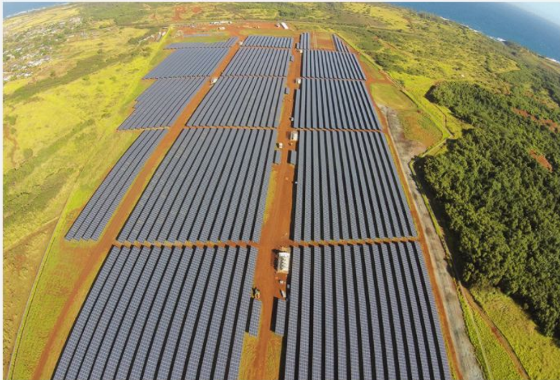
Kauai Island Utility Cooperative's Anahola Solar Farm, Kauai, Hawaii. 12 MW with a 6 MWh battery system. Scheduled to be operational in 2015. With this and other solar farms Kauai Island Utility Cooperative is proactive in reducing dependence on and costs of oil fired power plants. 12.5 cents/kWh (solar) versus 24 cents (oil).
