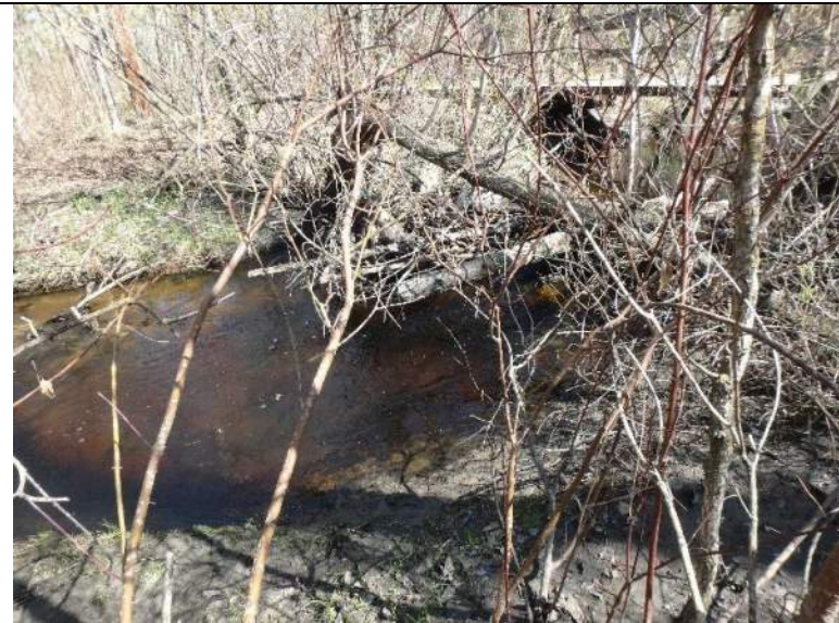
Plate 6: View upstream, showing large log jam at bridge B310
