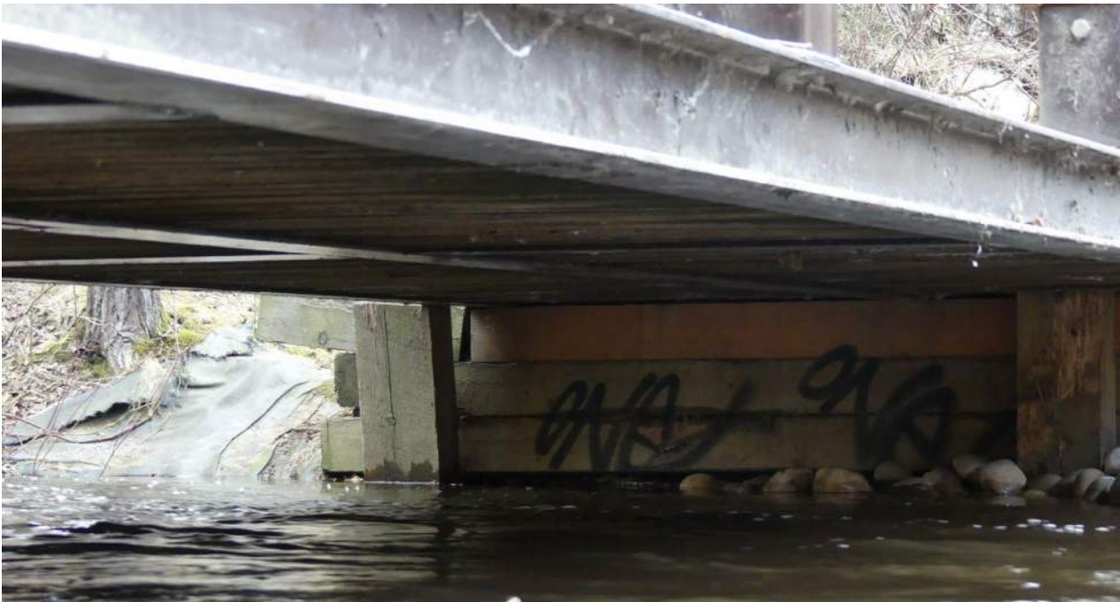
Photo B-2 (File No. P1000911) – Representative photograph of typical bridge underside. No evidence of cliff or barn swallow nesting was observed.
