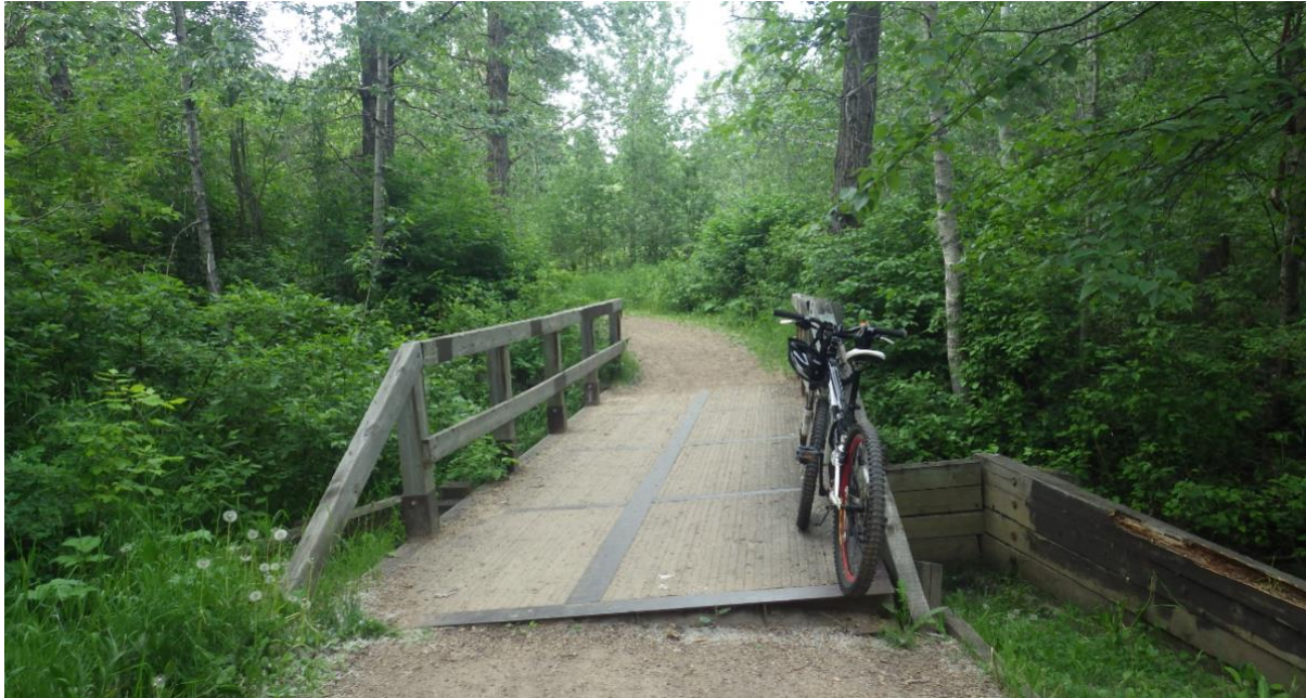
Figure 4.8.2: Bridge B309, Showing Visual Signs of Age and Deterioration (June 26, 2020).
