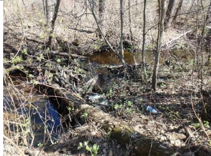
Plate 4: View upstream, approximately 100 m upstream of bridge B311 showing significant instream debris
