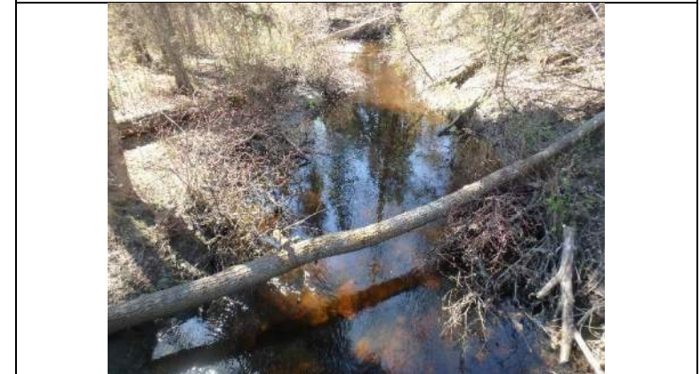
Plate 2: View upstream from bridge B311 showing run habitat, and rip rap present
