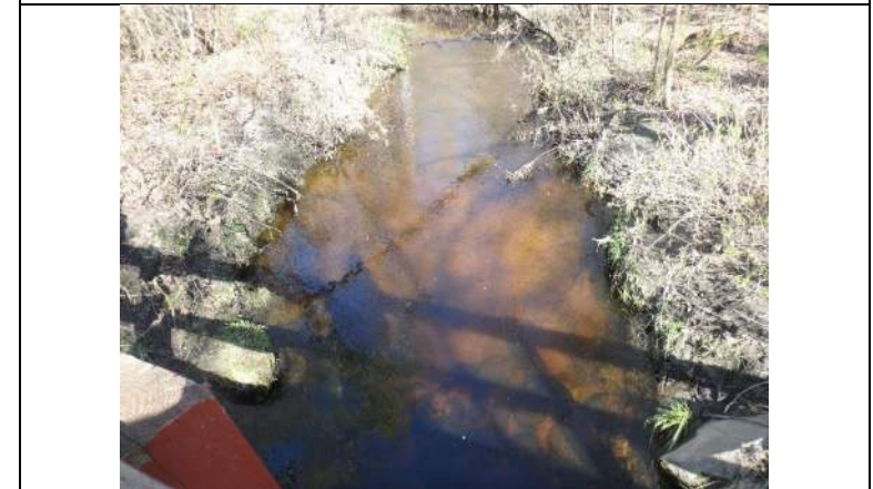
Plate 2: View upstream and under bridge B305, showing riprap present, and riffle upstream of site
