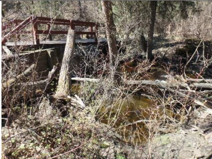
Plate 5: View upstream towards bridge B311, showing extensive instream debris
