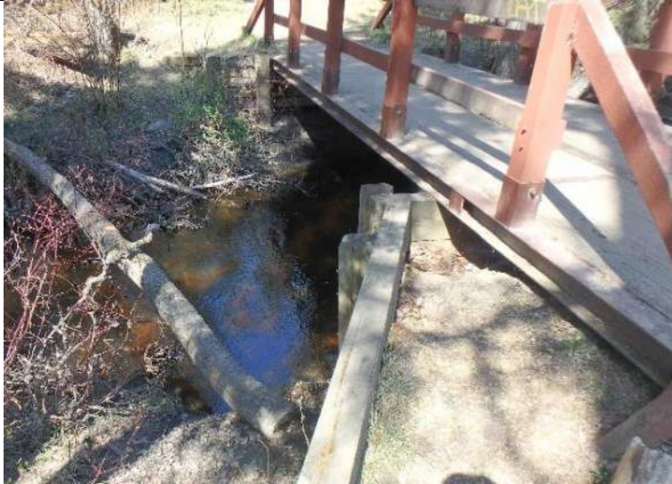
Plate 3: View across from bridge B311, showing erosion present
