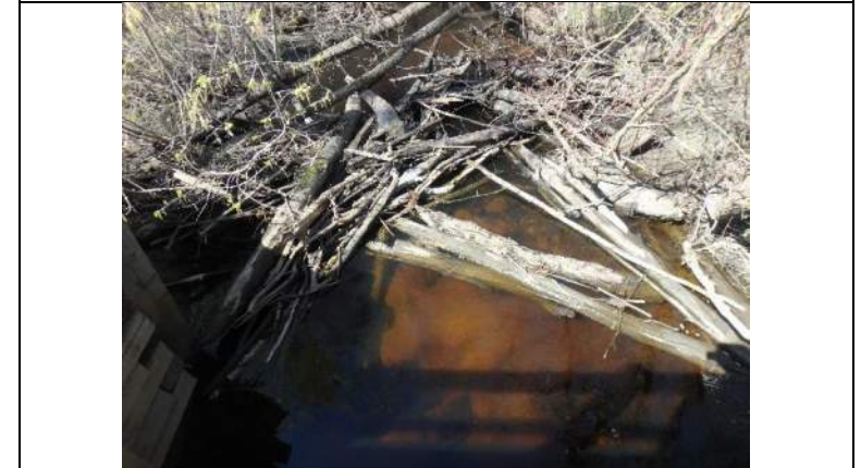
Plate 2: View downstream from bridge B310, showing extensive large woody debris and riprap presence
