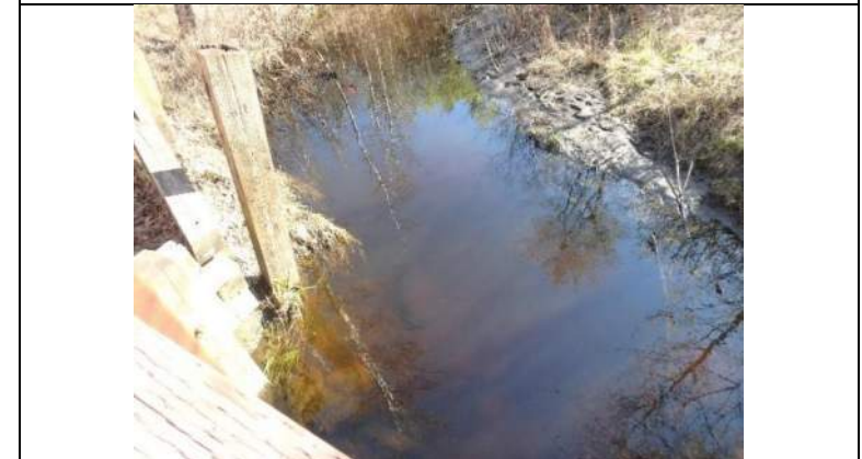
Plate 2: View upstream from bridge B304 showing silt and riprap
