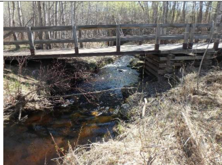
Plate 6: View downstream towards bridge B307 showing riffle downstream of bridge, and riprap present
