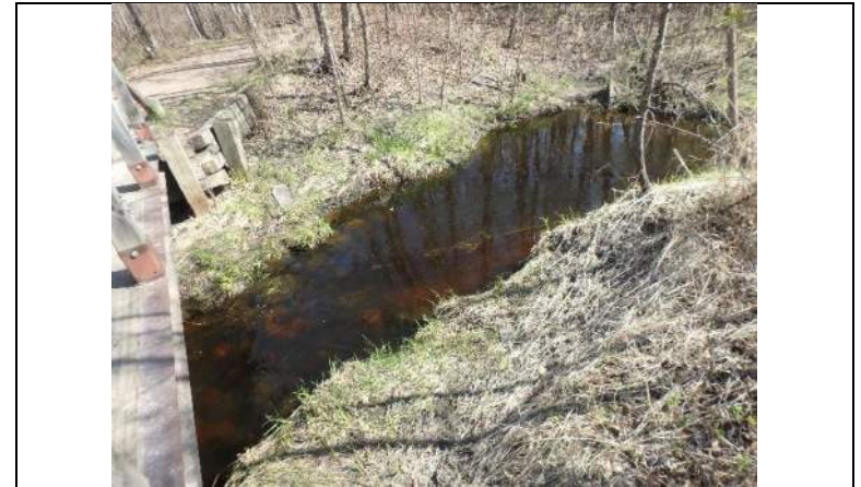
Plate 1: View upstream from bridge B306, showing riprap presence and shallow pool habitat
