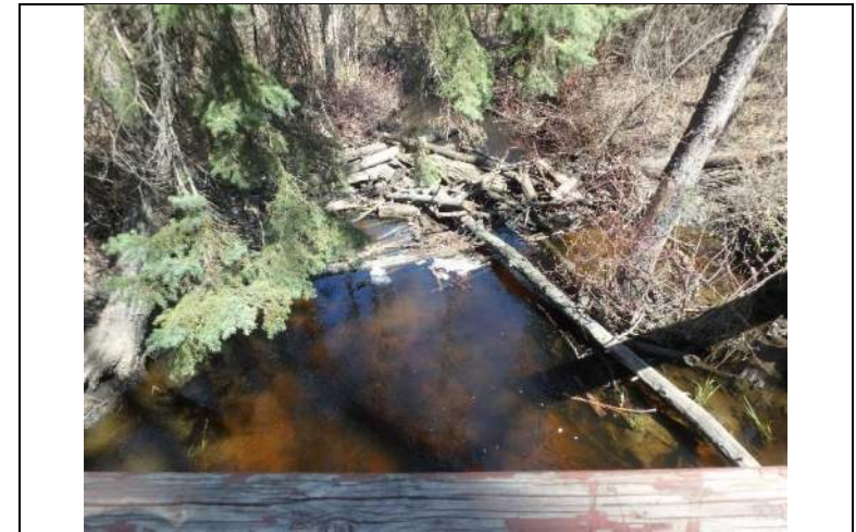
Plate 1: View downstream from bridge B311, showing significant large woody debris pile immediately downstream of bridge
