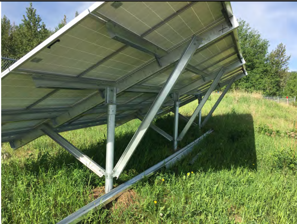
Plate 2: Demo racking currently on site
