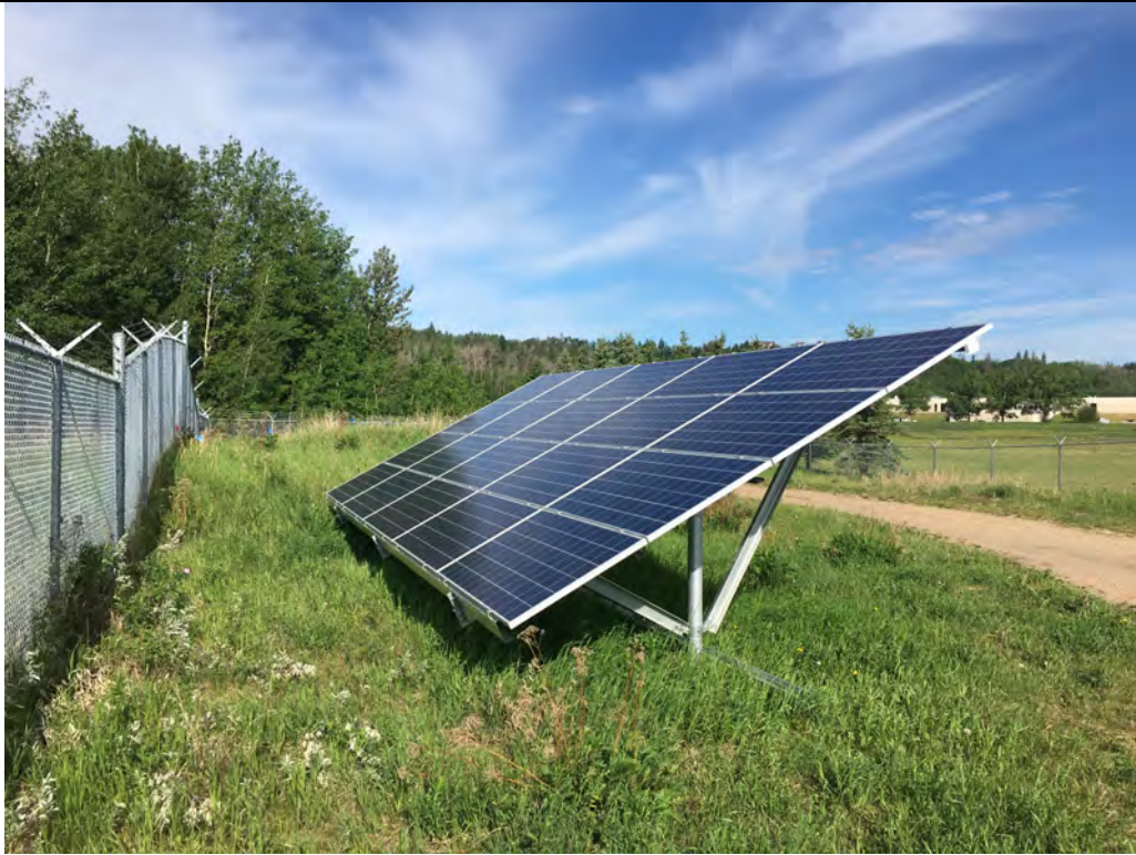
Plate 1: Demo solar panel currently on site
