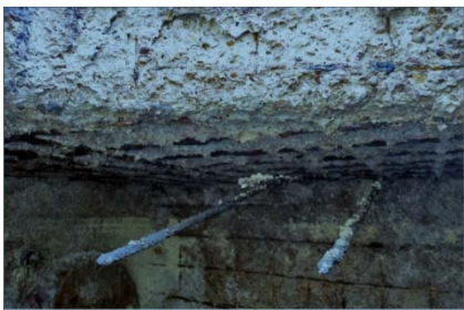
Rebar failure in Gold Bar Utilidor
