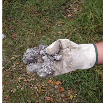
Handful of corroded concrete from manhole, Mill Creek
