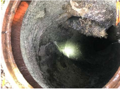
Corroded manhole, Mill Creek
