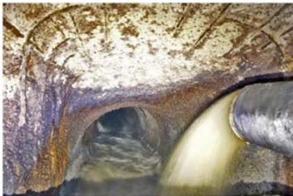
Sulfur deposits & exposed rebar from corrosion, Duggan Sanitary Tunnel
