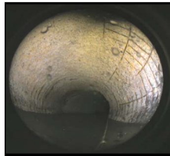
100 mm of concrete corrosion exposes rebar in Clareview Sanitary Trunk
