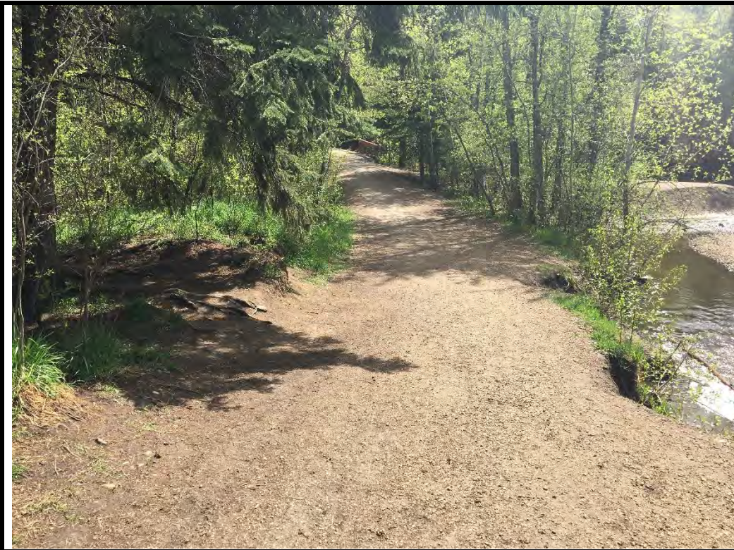
Photo 7: Site 3; eroded bank impacting trail at right of photo, intersection with single track trail at left of photo (facing south)
