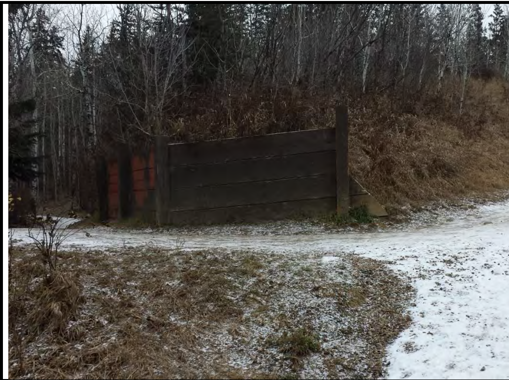
Photo 4: Site 2; existing retaining wall at toe of 5H:1V slope (facing northeast, taken November 19, 2016)
