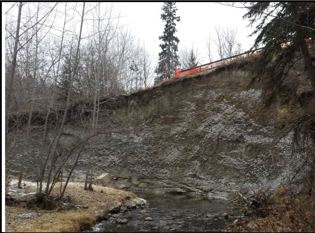
Photo 5: Site 2; eroding bank below trail (facing north, taken November 19, 2016)
