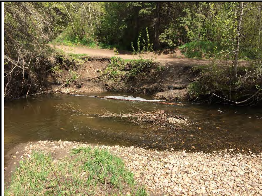
Photo 6: Site 3; eroded bank impacting trail (facing northeast)
