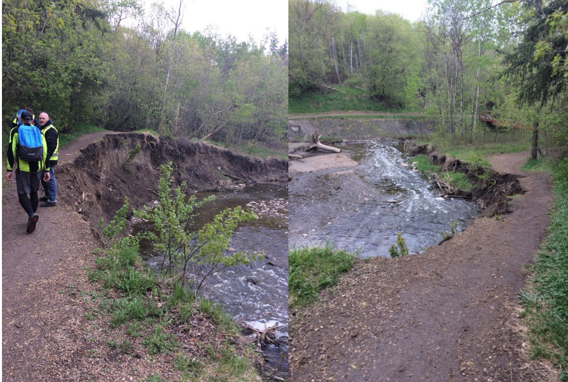
Figure 6 View of Site 1 trail eroding into creek - View looking south (left) and north (right).
