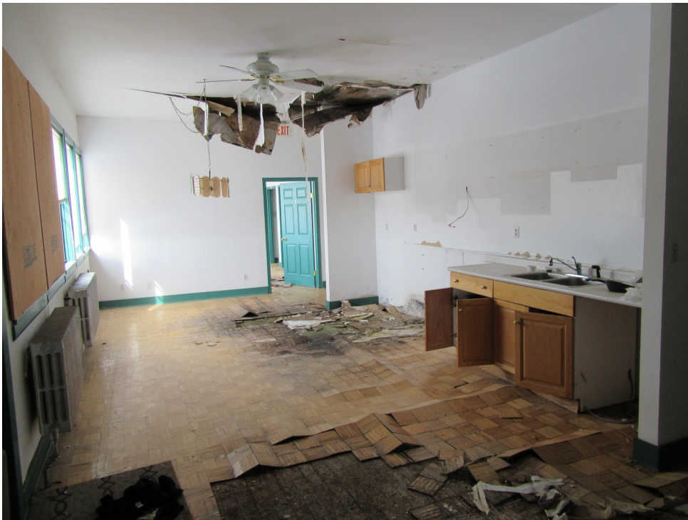
Detail showing typical conditions of spaces within the office wings on the east and west elevations of Hangar 11.
