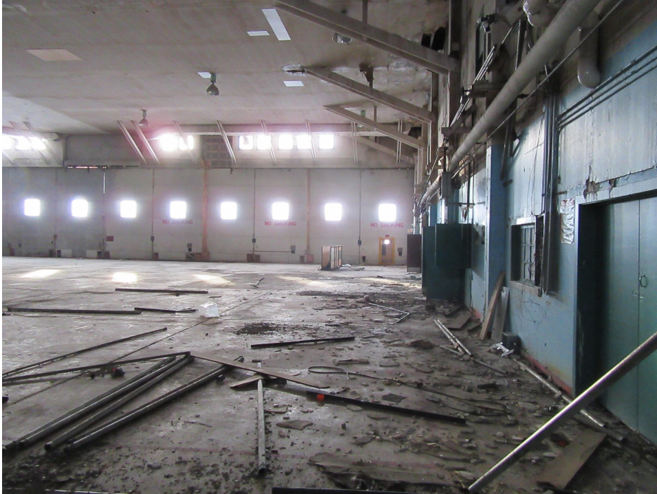
Interior view of main hangar space, looking south from northwest corner of hangar.
