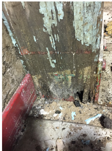
Photo 5: Damaged Column – Hole at Bottom where screwdriver could go in
