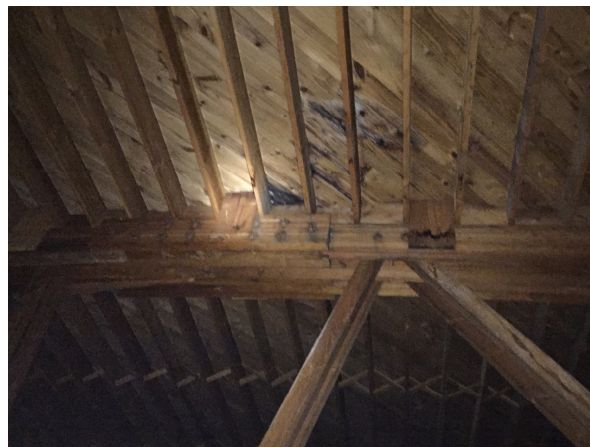
Photo 1: Truss top – signs of water infiltration
