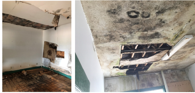
Photos 8 to 9: Ancillary Framing – Damaged Finishes due to water Infiltration
