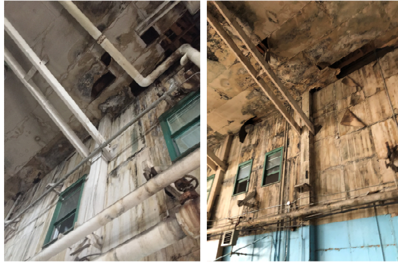
Photos 3 and 4: Hanger Walls – Signs of Deterioration
